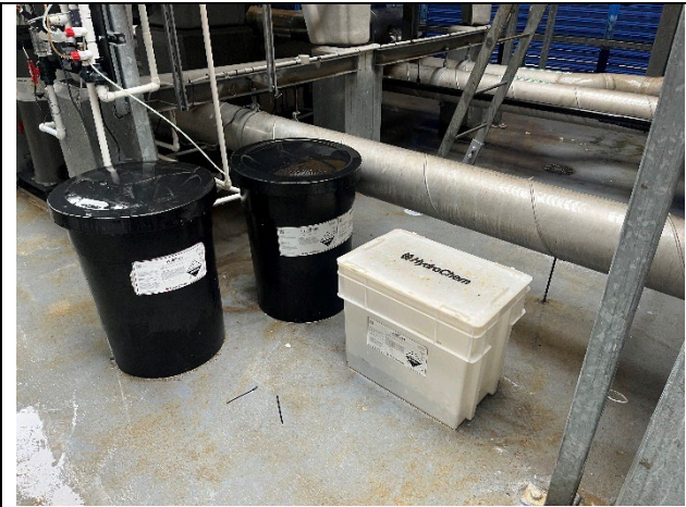
Photo 01. Level 33 Cooling Tower Chemicals – incorrect label on secondary containment.
