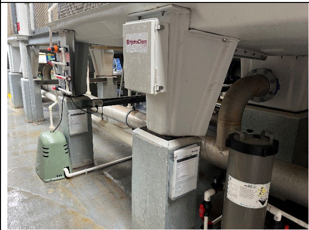
Photo 03. SDS's in the Level 33 Cooling Tower Area.
