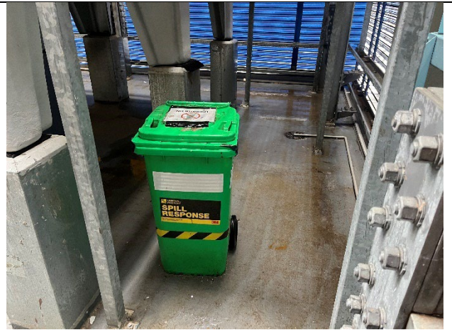
Photo 02. Spill kit in the Level 33 Cooling Tower Area.
