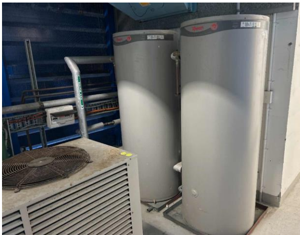
Line ID 12.1: Internal, L19, Plant Room, Hot Water Heater, Insulation Material - Suspected SMF
