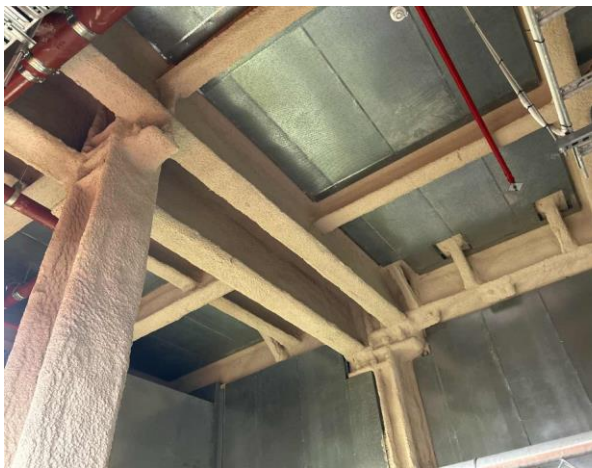
Line ID 3: Internal, All Levels, Throughout, Sprayed Coating to Beams, Ductwork and Pipework., Sprayed Vermiculite - No Asbestos Detected
