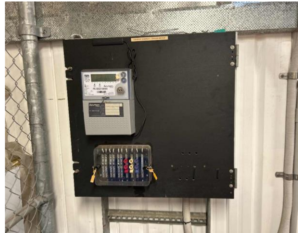
Line ID 2: Internal, All Levels, Throughout, Electrical Switchboards, Bituminous Backing Board - No Asbestos Suspected
