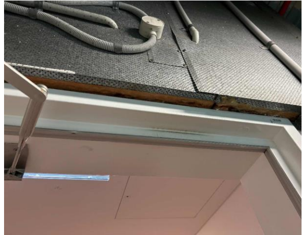
Line ID 8.1: Internal, All Levels, Throughout, Metal Cased SMF Cladding to Doors, Ceilings & Walls, Insulation Material - Suspected SMF
