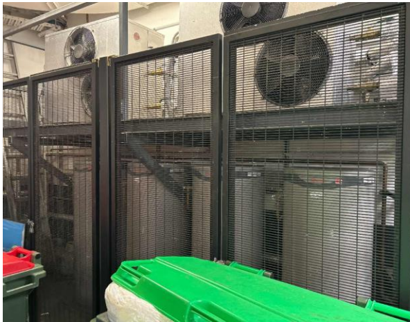
Line ID 11: Internal, B1, Loading Dock, Hot Water Heaters, Insulation Material - Suspected SMF
