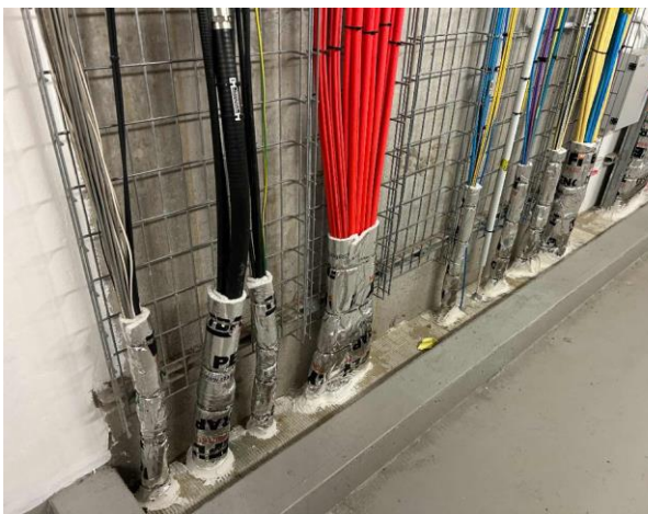
Line ID 10.1: Internal, All Levels, Throughout, Pipework Insulation to Walls and Ceilings, Insulation Material - Suspected SMF
