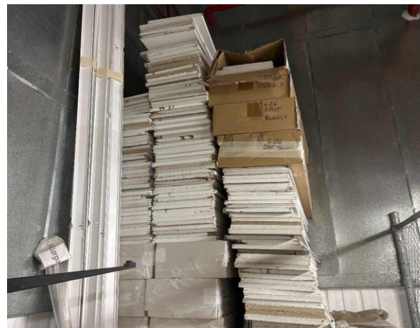
Line ID 14.1: Internal, L32, Plant Room, Southwest Corner, Storage Cage, Compressed Ceiling Tiles - Suspected SMF
