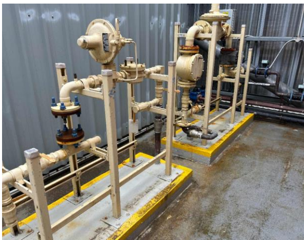
Line ID 6: External, L33, Throughout, Gas Supply Pipework, Beige Paint - Lead Detected (0.02% w/w)
