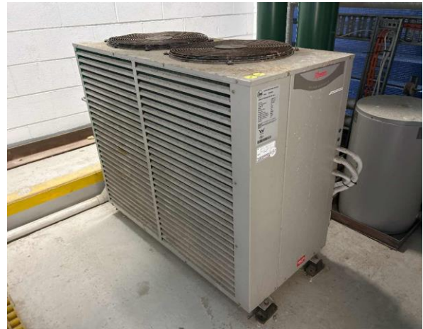
Line ID 16: Internal, L19, Plant Room, Hot Water Heater Pump, R407C Hydrofluorocarbon (HFC) - Non ODS Refrigerant
