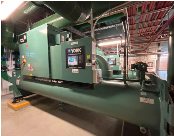
Line ID 17: Internal, L31, Plant Room, Centrifugal Chillers, R134a Hydrofluorocarbon (HFC) - Non ODS Refrigerant
