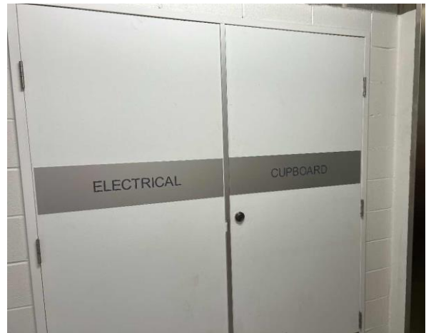
Line ID 21: Internal, L20, Electrical Cupboard – No Access
