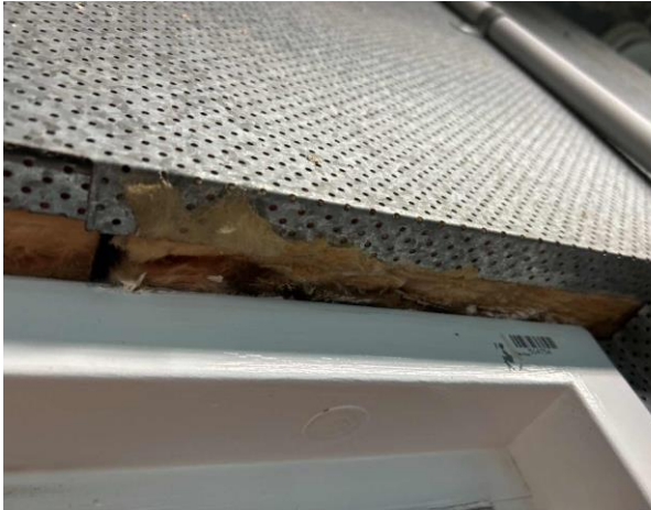
Line ID 8: Internal, All Levels, Throughout, Metal Cased SMF Cladding to Doors, Ceilings & Walls, Insulation Material - Suspected SMF
