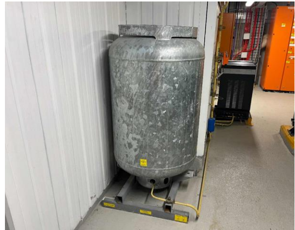
Line ID 18: Internal, L31, Plant Room, Spare Tank, R134a Hydrofluorocarbon (HFC) - Non ODS Refrigerant
