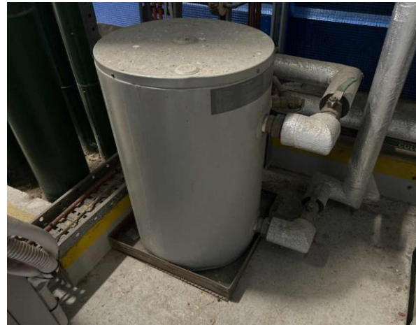
Line ID 12: Internal, L19, Plant Room, Hot Water Heater, Insulation Material - Suspected SMF
