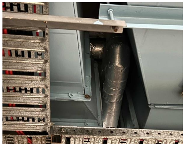
Line ID 10.2: Internal, All Levels, Throughout, Pipework Insulation to Walls and Ceilings, Insulation Material - Suspected SMF
