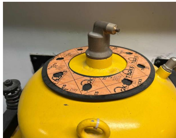
Line ID 4: Internal, L30, Plant Room, Gasket on top of Water Condenser, Gasket Material - No Asbestos Detected
