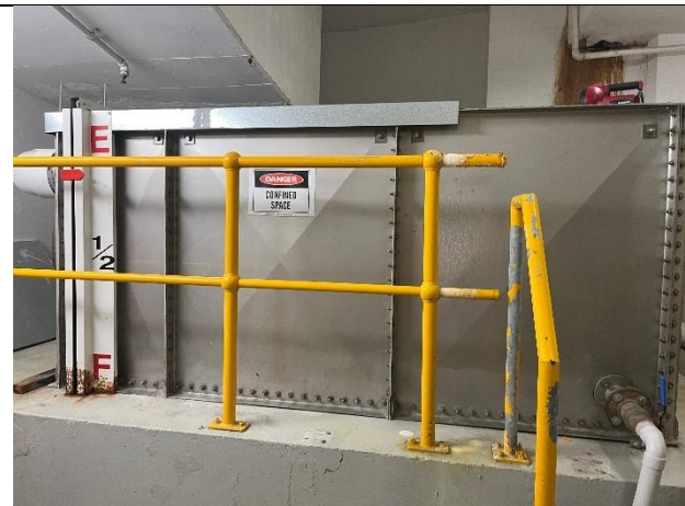
Photo 17. Level B2, Stormwater Pump Room, water tank.
