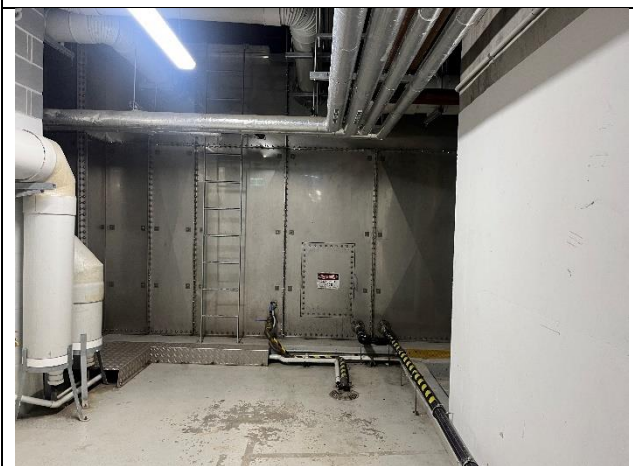
Photo 05. Level 4 Plant Room, water tank.
