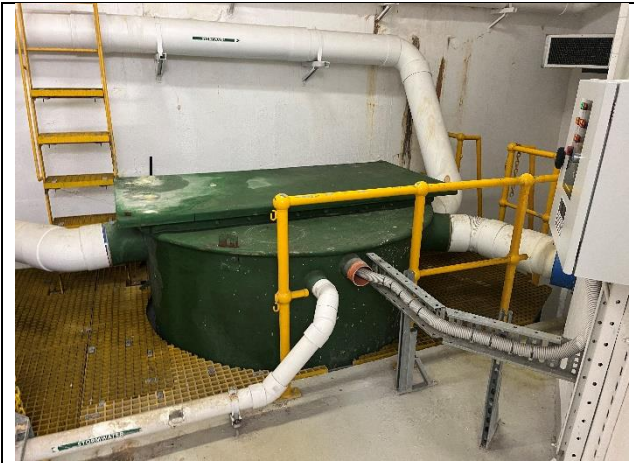
Photo 19. Level B2, Stormwater Pump Room, sump pump pits x 2.
