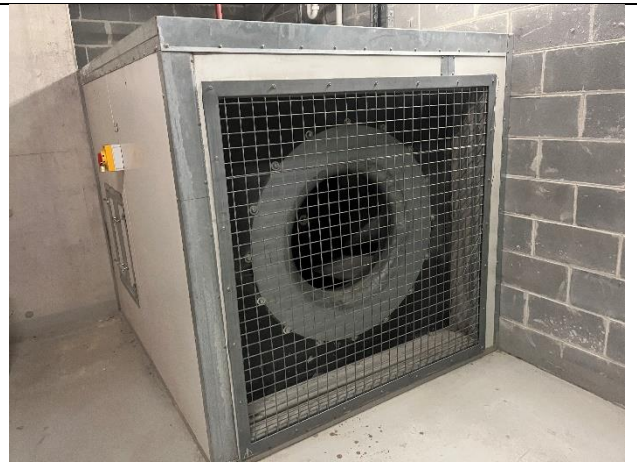
Photo 16. Level B2, Plant Room, carpark exhaust fan chamber.
