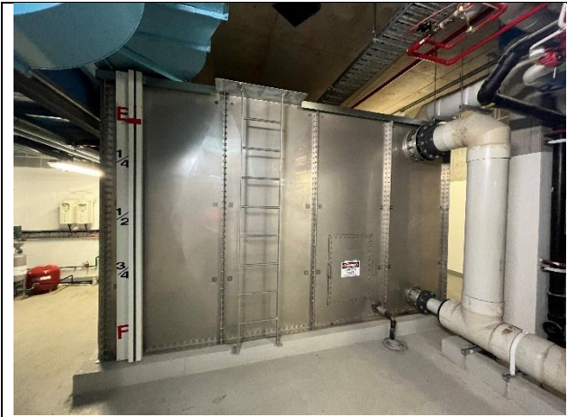
Photo 07. Level 3 Plant Room, water tank.
