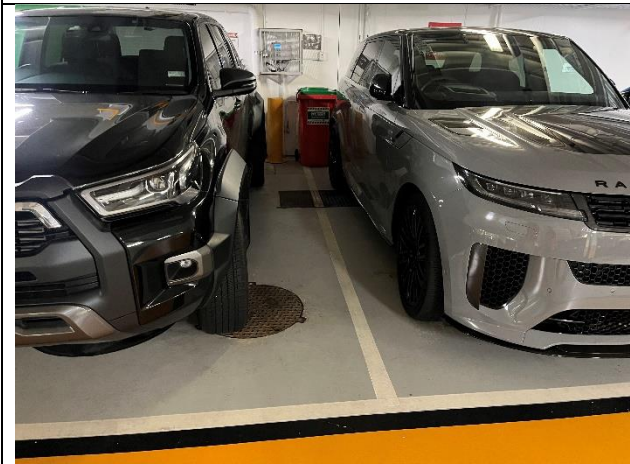
Photo 09. Level B2, carpark, adjacent spaces 15 and 16, grease traps x 2.
