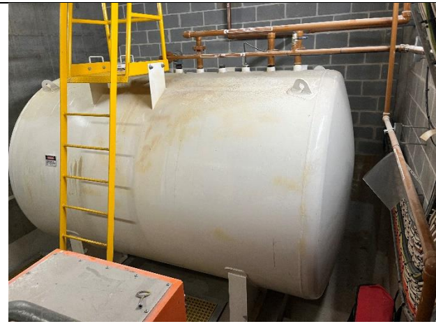
Photo 15. Level B2, Diesel Tank Room, diesel tank.
