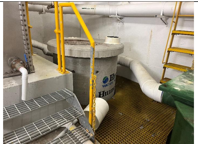
Photo 18. Level B2, Stormwater Pump Room, sump pump pits x 2.
