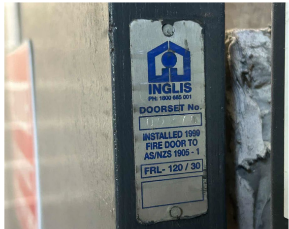
Line ID 2.1: Internal, All Levels, Stairwells and Plant Rooms, Various Throughout, Fire Door Core - No Asbestos Detected
