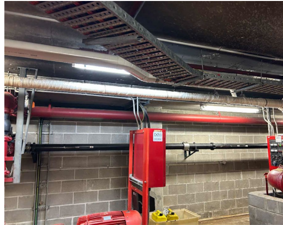
Line ID 16: Internal, B4, Hydrant Pump Room, Pump Exhaust Pipes, Insulation Material - Suspected SMF
