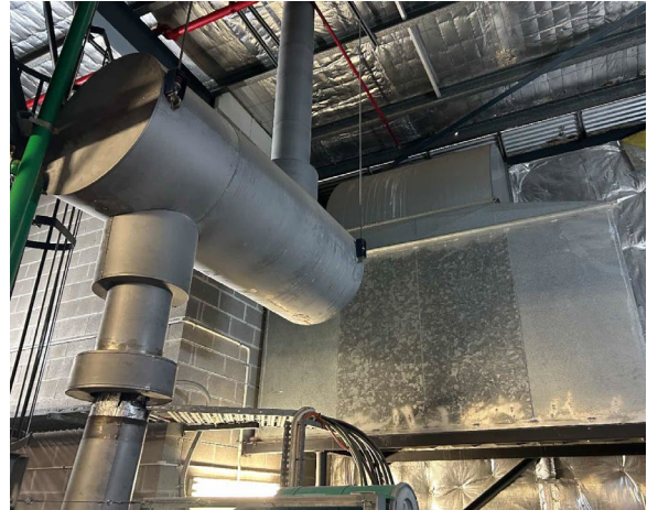
Line ID 26: Internal, L15, Generator Room, Generator Exhaust and Acoustic Baffles, Insulation Material - Suspected SMF
