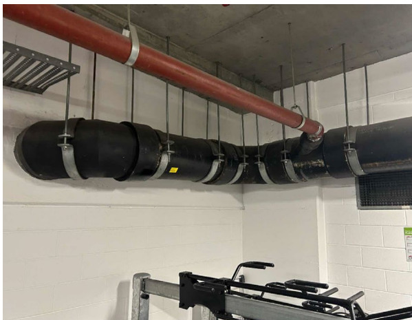
Line ID 3: Internal, B1, Carpark and End of Trip Room, Black Stormwater Pipework, Moulded Fibre Cement - No Asbestos Detected
