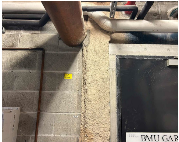
Line ID 7: Internal, L15, Chiller Room, Structural Beams, Sprayed Vermiculite - No Asbestos Detected
