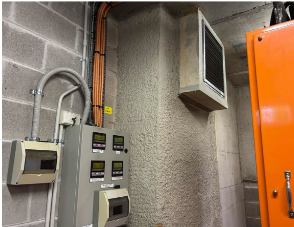
Line ID 6: Internal, B1, Main Switch Room, Ductwork, Sprayed Vermiculite - No Asbestos Detected
