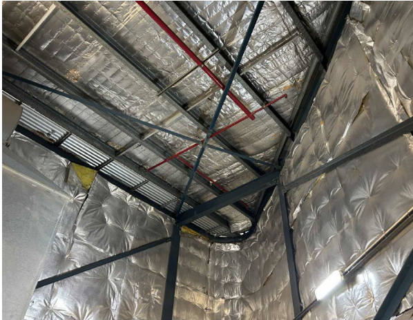
Line ID 25: Internal, L15, Generator Room, Ceiling and Walls, Sarking Insulation - Suspected SMF
