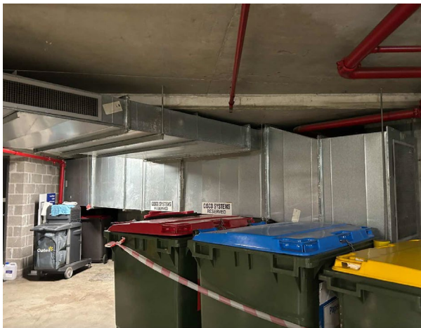
Line ID 17: Internal, B4-B1, Carpark, Ductwork, Internal Lining, Insulation Material - Suspected SMF
