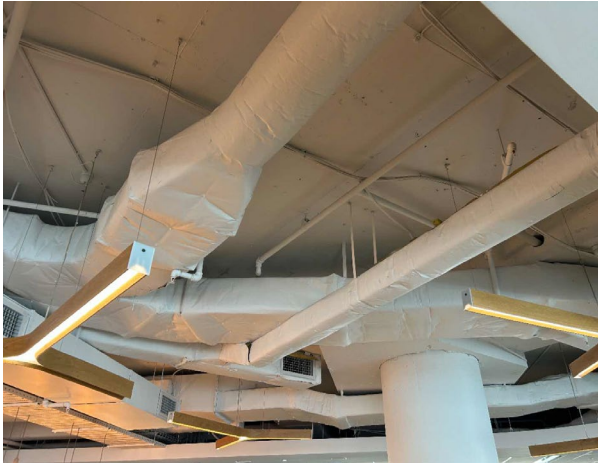
Line ID 19: Internal, L1-14, Office Areas, Ceiling Space, Ductwork, Insulation Material - Suspected SMF
