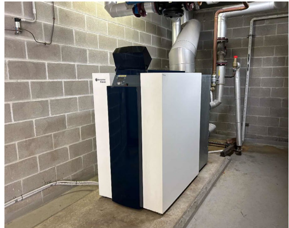
Line ID 22: Internal, L15, Boiler Room, Boiler and Pipework, Insulation Material - Suspected SMF
