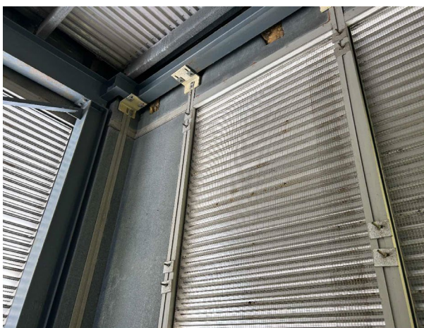
Line ID 11: Internal, L16, Cooling Tower Room, Within Metal Wall Cladding, Insulation Batts - Suspected SMF
