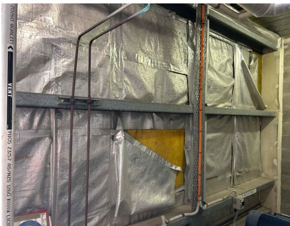
Line ID 23: Internal, L15, Boiler Room, Wall, Sarking Insulation - Suspected SMF
