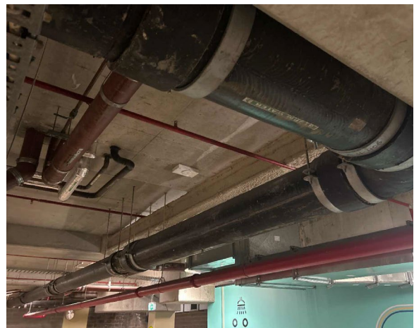
Line ID 3.1: Internal, B1, Carpark and End of Trip Room, Black Stormwater Pipework, Moulded Fibre Cement - No Asbestos Detected
