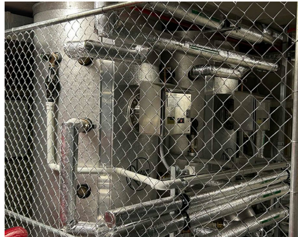
Line ID 14: Internal, B3, Carpark, Caged Area, Water Heaters, Insulation Material - Suspected SMF
