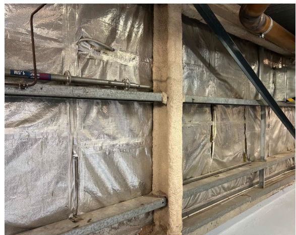
Line ID 24: Internal, L15, Chiller Room, Wall, Sarking Insulation - Suspected SMF
