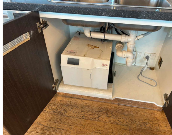
Line ID 20: Internal, L1-14, Office Areas, Kitchenettes, Water Heaters, Insulation Material - Suspected SMF
