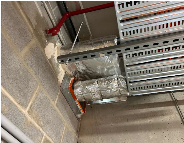
Line ID 13: Internal, All Levels, Plant, Service and Electrical Areas, Various Areas, Foil Lined Insulation to Pipework and Cables, Insulation Material - Suspected SMF
