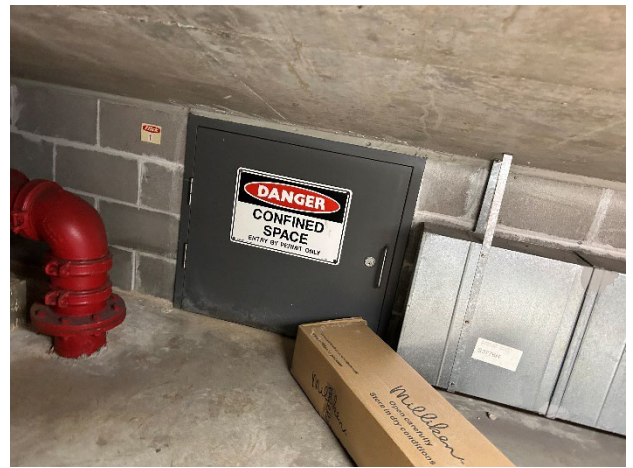
Photo 06. Level B4, car park, adjacent to lift lobby – void.
