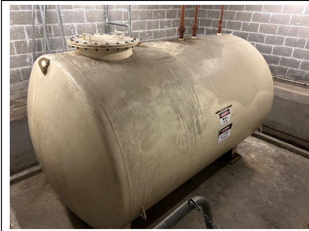
Photo 01. Diesel Tank Room – fuel tank.
