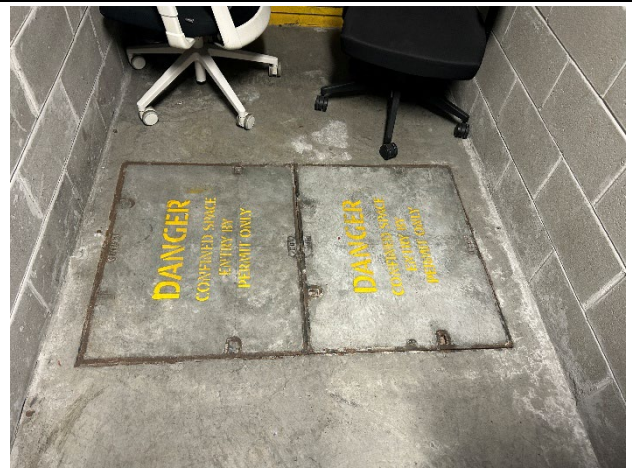
Photo 08. Level B3, corridor adjacent to the Fan Room – unknown pit.
