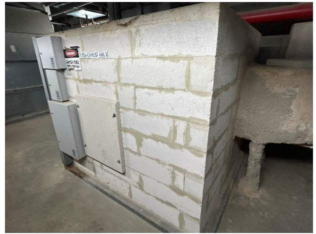
Photo 10. Level 15, AHU Room – exhaust fan chamber.
