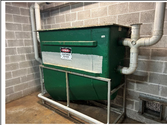
Photo 07. Level B3, Grease Arrestor Room – grease trap.
