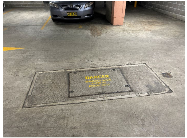
Photo 04. Level B4, car park, adjacent to parking space 2 – unknown pit.
