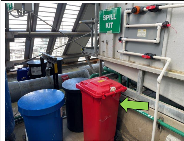
Spill kit available in the Cooling Tower Area
