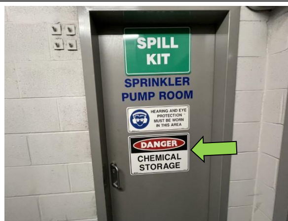
Hazard chemical warning signage was installed at the entrance to the Sprinkler Pump Room
