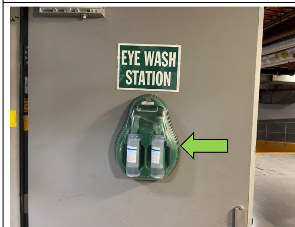
Eye wash station available in the Cleaners Store Room
