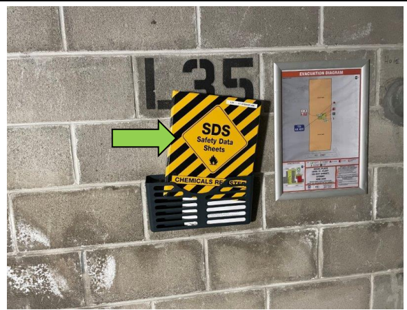
Current SDS's were available for the cooling tower chemicals
