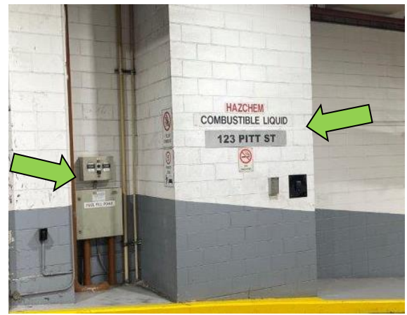
Placarding installed at main vehicle entrance to the site and diesel fill point
