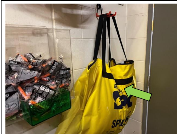
Spill kits available in the Sprinkler Pump Room
