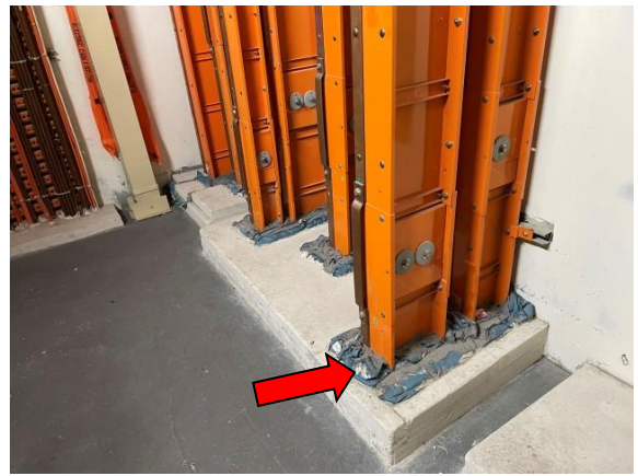
Photo 10: All Levels, Electrical penetrations – SMF pillow insulation
