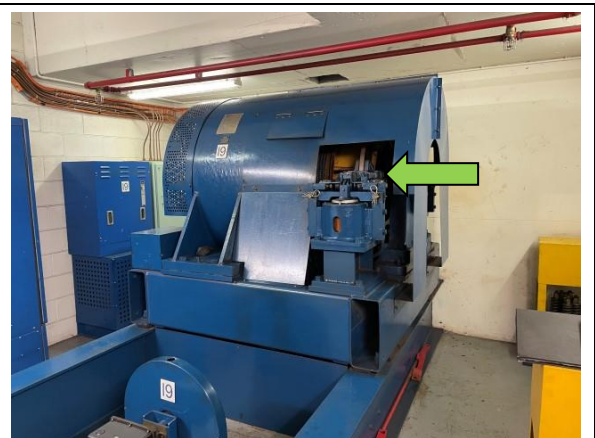
Photo 2: Level 32, High Rise Lift Motor Room, Lift Motor – Non-asbestos brake pads
