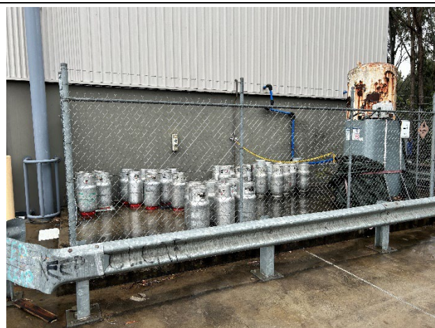
Photo 04. LPG storage area on northwest side of Building 1.
