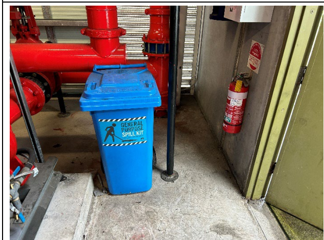
Photo 03. Spill kit and fire extinguisher in Building 2 Fire Pump Room.
