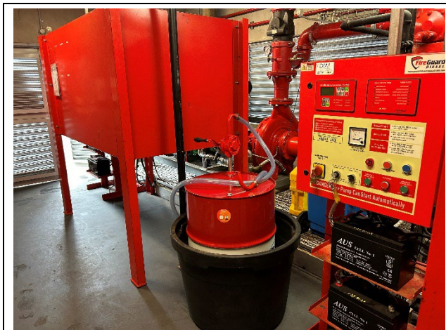
Photo 01. Hazardous chemical storage within the Building 4 Fire Pump Room.
