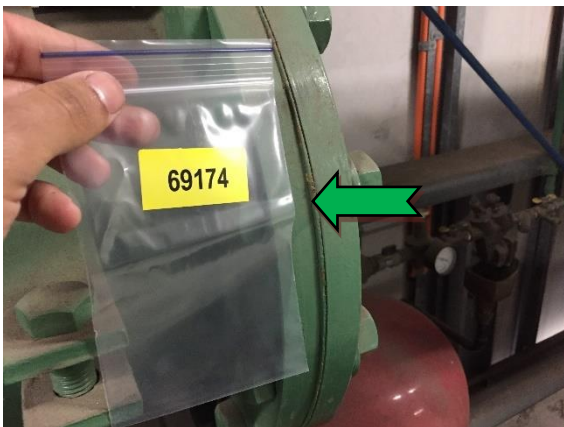
Photo 5 Interior: level 16, plant room, pump machinery – non-asbestos containing gasket material.
