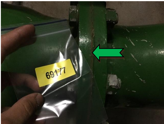
Photo 9 Interior: level 16, plant room, York chiller – non-asbestos containing gasket material.
