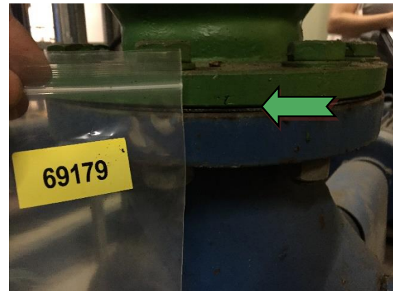
Photo 12 Interior: level 16, plant room, pump adjacent York chiller – non-asbestos containing gasket material.
