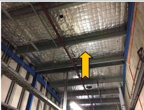
Photo 17 Interior: level 16, plant room, ceiling – suspected SMF containing sarking insulation.
