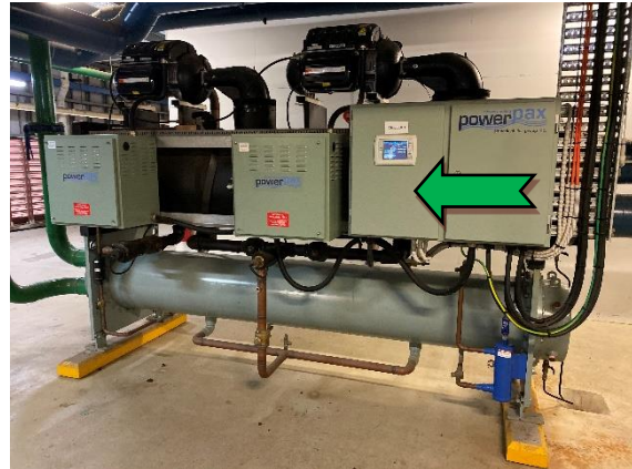
Photo 22 Interior: level 16, plant room, Power Pax chiller – non-ODS containing R134a hydrofluorocarbon refrigerant.
