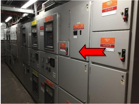
Photo 1 Interior: carpark level 8, main switch room, switchboard – suspected asbestos containing fuses.
