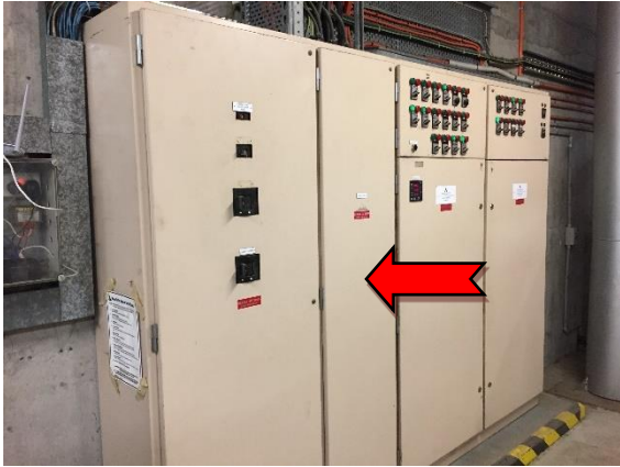
Photo 7 Interior: level 16, plant room, switchboard – suspected asbestos containing fuses.
