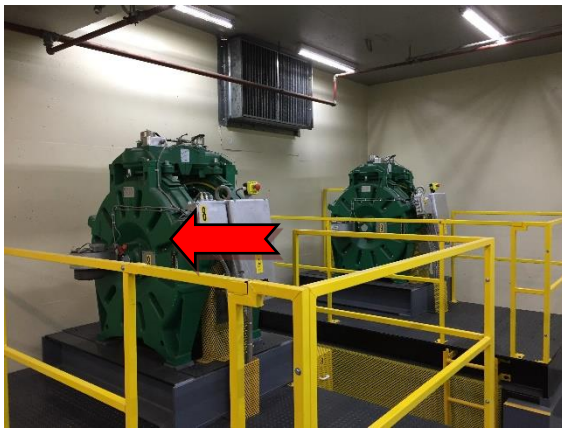
Photo 15 Interior: lift motor room, lift motor – suspected asbestos containing friction pads.
