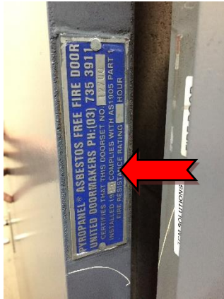
Photo 13 Interior: all levels, throughout, fire doors – suspected asbestos containing fire door core.
