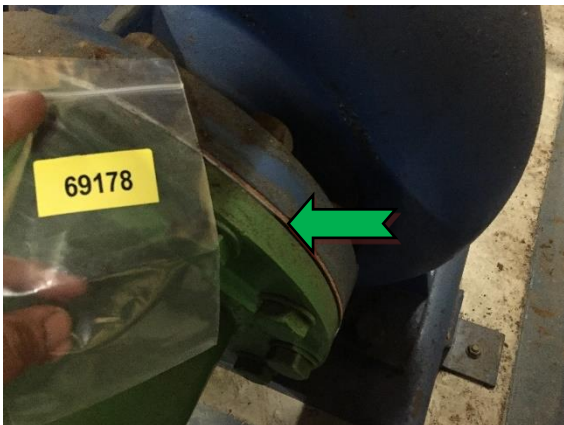
Photo 11 Interior: level 16, plant room, pump adjacent York chiller – non-asbestos containing gasket material.
