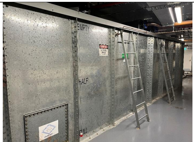
Photo 04. L4, Tank Room, DCW buffer tank #1.
