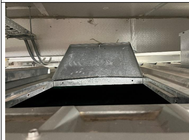
Photo 05. L4, Tank Room, DCW buffer tank #1, lid open
