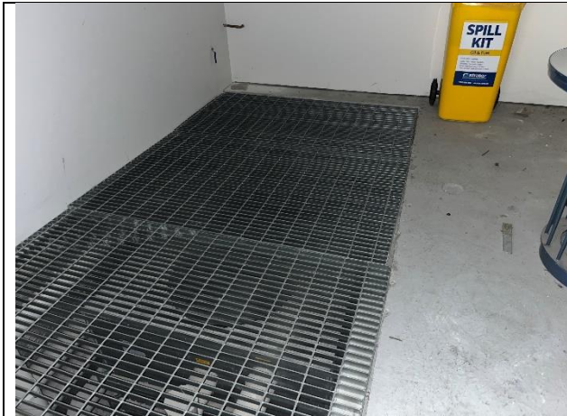
Photo 01. L2, Grease Trap Room, grease trap.
