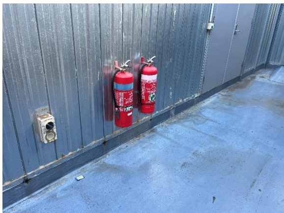
Photo 03. Fire extinguishers adjacent to diesel storage in Level 13 Cooling Tower Area.
