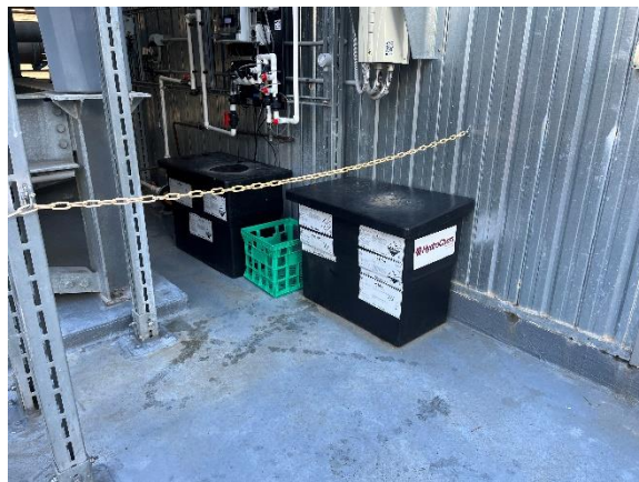
Photo 02. Chemical storage in Level 13 Cooling Tower Area.
