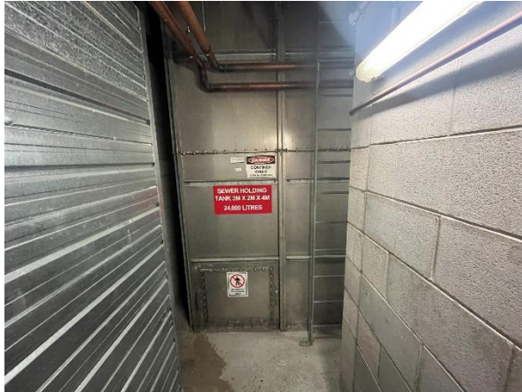
Photo 01. L3, Sewer Holding Tank Room, sewer tank.
