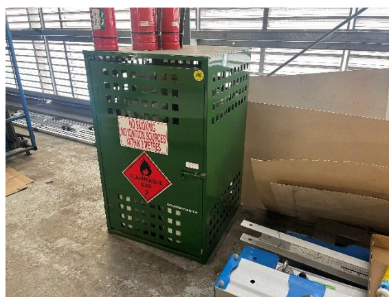
Photo 04. LPG storage in Level 12 Plant Room.
