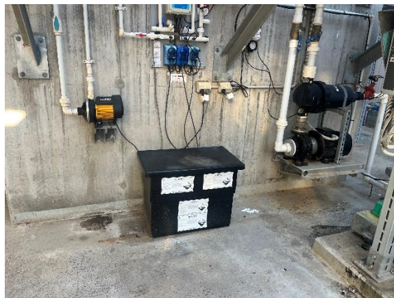
Photo 02. Chemical storage in Level 12 Cooling Tower Area.
