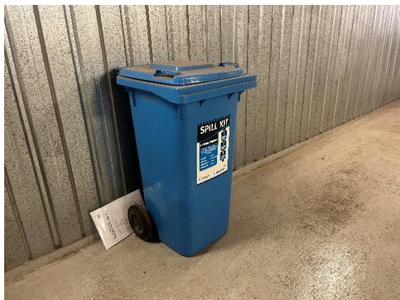
Photo 01. Spill kit in Level 12 Plant Room.
