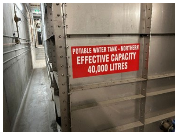
Photo 04. Level 1 Fire Tank Room Northern, Potable Water Tank
