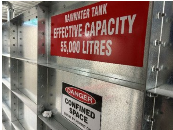
Photo 01. Level 3 Plant Room, RW Tank
