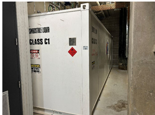
Photo 10. Ground Floor Loading Dock, Fuel Area, 19,000L Diesel Tank.
