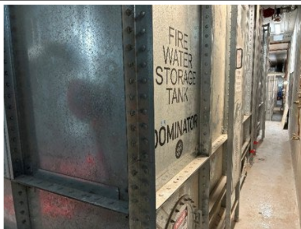
Photo 03. Level 1 Fire Tank Room, Fire Tank
