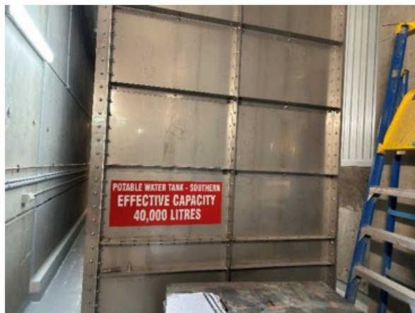
Photo 05. Level 1 Fire Tank Room Southern, Potable Water Tank
