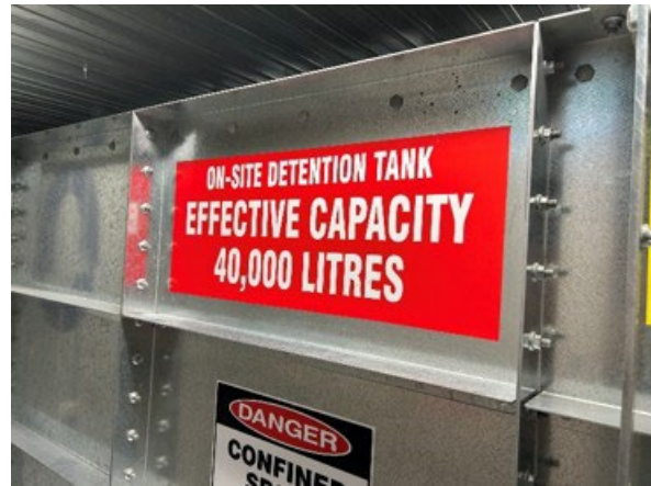
Photo 02. Level 3 Plant Room, OSD Tank
