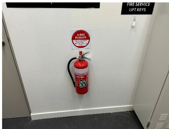
Photo 14. Ground Floor Fire Pump Room ABE fire extinguisher.
