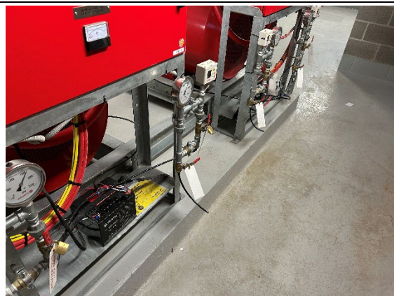
Photo 06. Level 1 Fire Pump Room 12v batteries.
