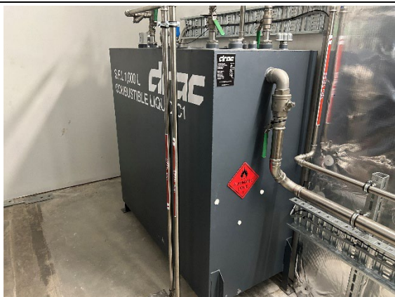
Photo 05. Level 21 Generator Room fuel tank.
