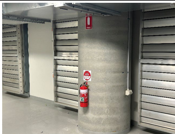
Photo 10. Fire extinguisher in the Level 10 Plant Room..
