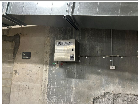
Photo 16. Ground Floor Loading Dock – Diesel Area, 19,000L Diesel Tank remote fill point.
