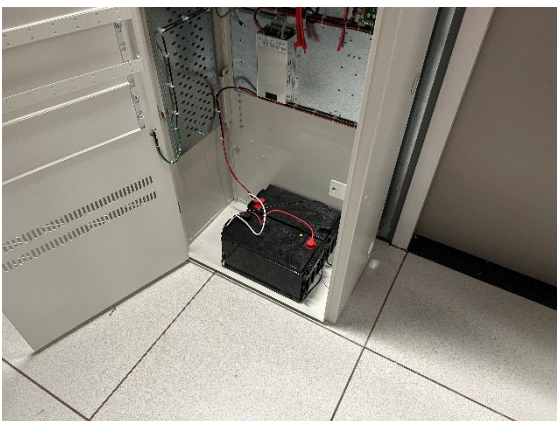
Photo 11. 12V Batteries in the Level 11 Electrical Riser Room Control Panel.
