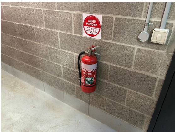
Photo 07. Level 1 Fire Pump Room ABE fire extinguisher.
