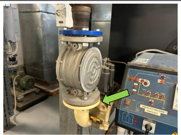
Photo 2: Level 15, Plant Room, Boiler Room, Pipework to Boiler – Non-asbestos containing gaskets
