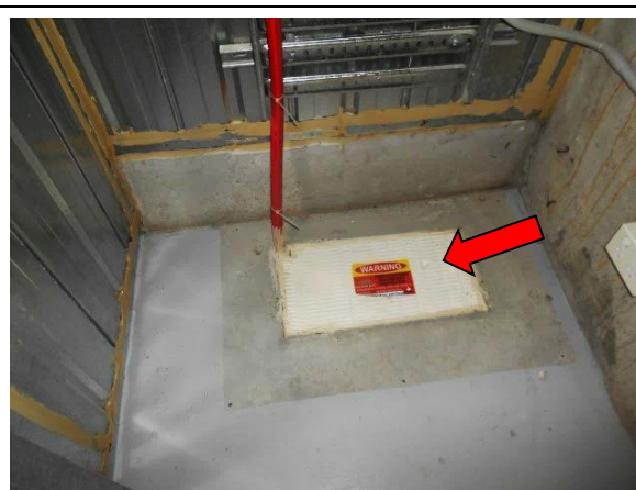
Photo 8: Office Levels, Electrical and Communications Cupboards – Fire stopping insulation to floor/ceiling penetrations
