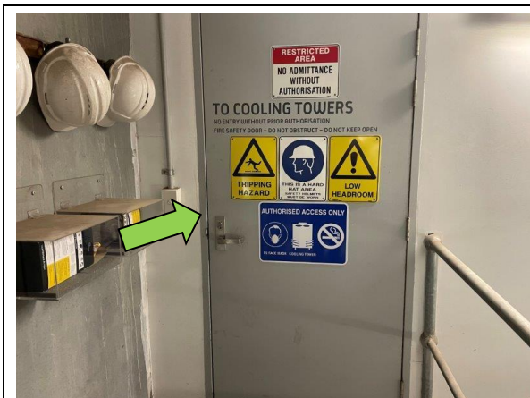
Cooling Tower Area appropriately signposted
