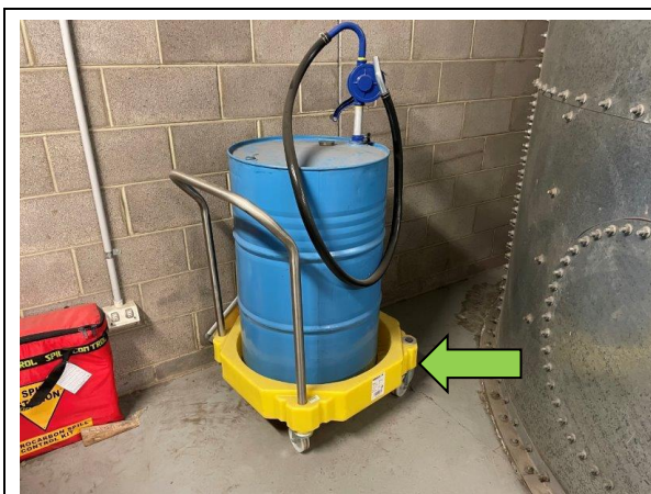
Appropriate secondary containment (bund) for the diesel fuel
