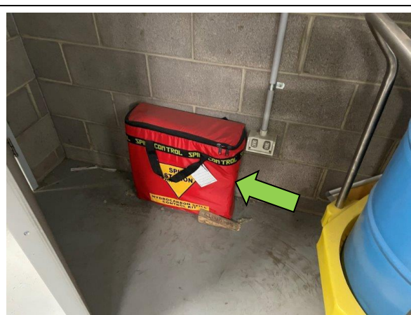
Spill kit available in the Fire Pump Room
