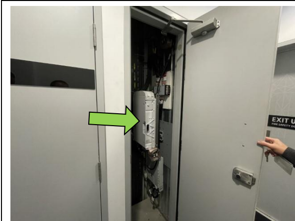
Communications cupboards located on levels housing the IBC system. (Note: no access controls required at the site)
