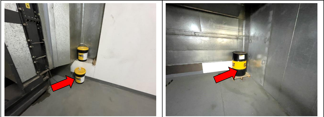
Hazardous chemicals were not stored in appropriate bunding
