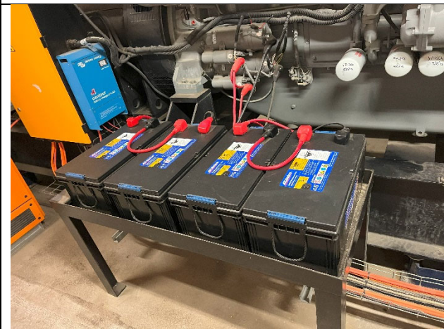
Photo 09. Level 18, Batteries adjacent the generator.
