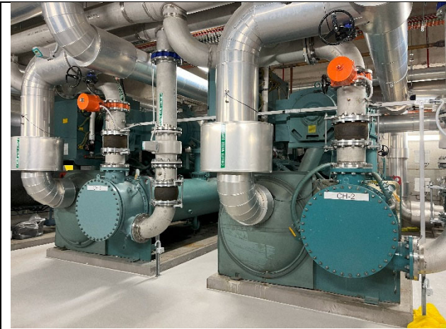
Photo 07. Level 18 Chiller Room.
