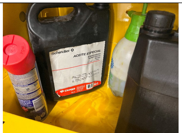
Photo 06. Spilled liquid in the base of the Level 17 Lift Motor Room Flammable Liquids Cabinet.
