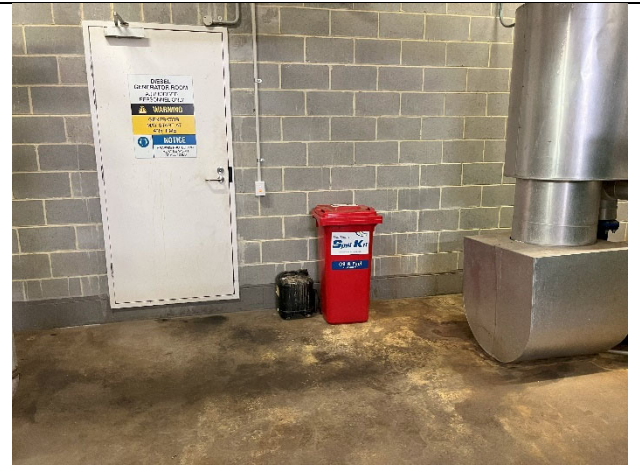
Photo 08. Level 18, spill kit adjacent the diesel generator room.
