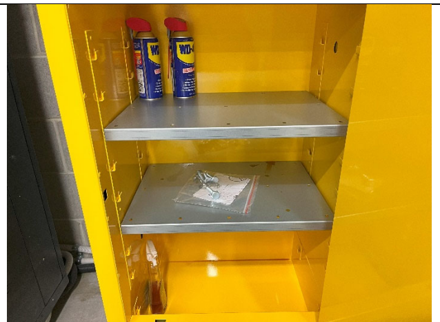
Photo 04. Class 2.1 Aerosols and Class 8 Corrosive chemicals stored within the Flammable liquids Cupboard in the Level 32 Lift Motor Room.
