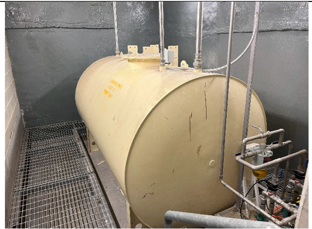
Photo 14. Basement level, diesel tank.
