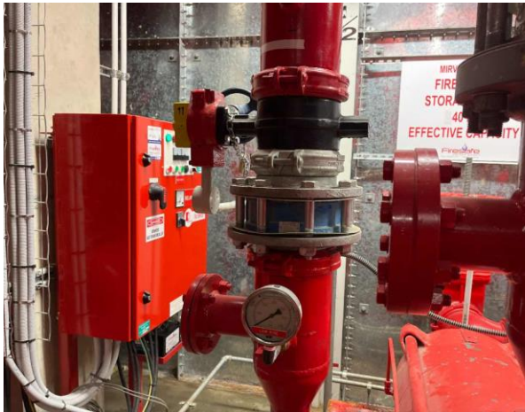
Line ID 7: Internal, Basement, Sprinkler Pump Room, White Gasket to Pumps, Gasket Material - No Asbestos Detected
