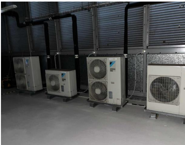
Line ID 27: Internal, L1, Plant Room, Daikin AC units, R410A Hydrofluorocarbon (HFC) - Non ODS Refrigerant
