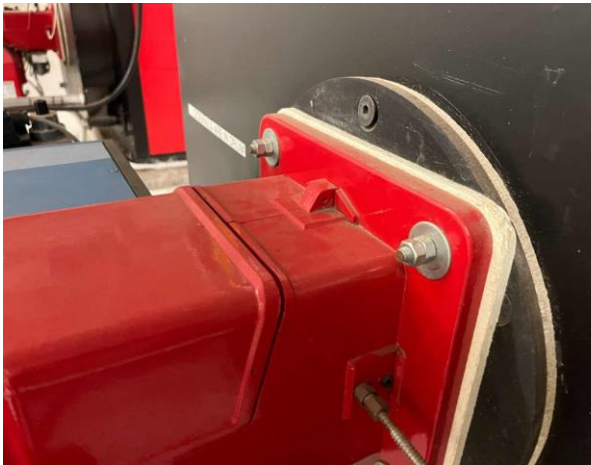
Line ID 3: Internal, L32, Plant Room, Boiler Room, Square Gasket to Boiler, Gasket Material - No Asbestos Detected
