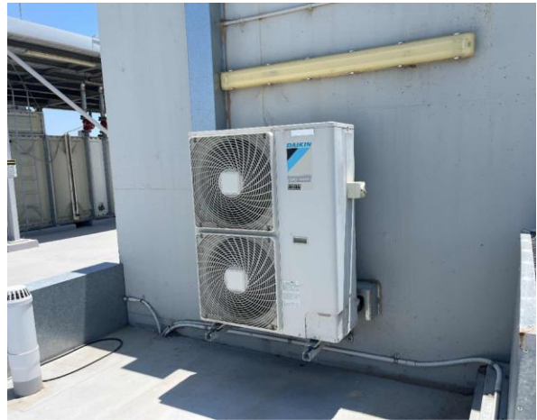
Line ID 26: External, Roof, East Side, Daikin AC Unit, R410A Hydrofluorocarbon (HFC) - Non ODS Refrigerant
