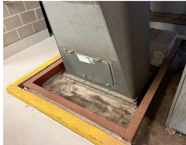
Line ID 10: Internal, L32, Plant Room, Floor at Base of AC Unit, Dust - Lead Detected (33mg/kg)
