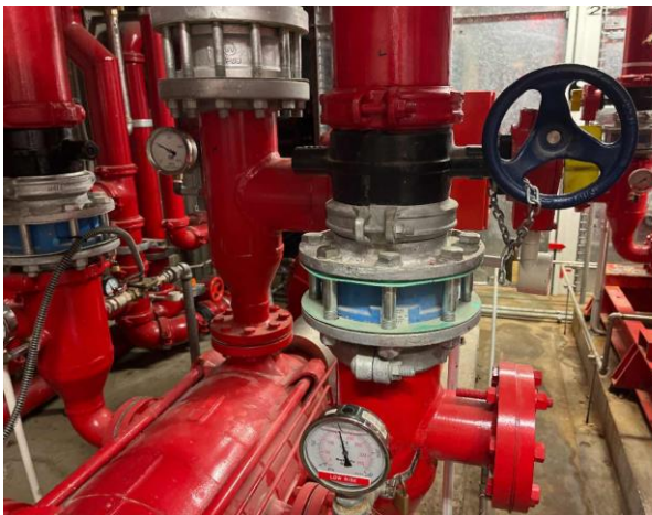
Line ID 5: Internal, Basement, Sprinkler Pump Room, Green Gaskets to Pipework, Gasket Material - No Asbestos Detected
