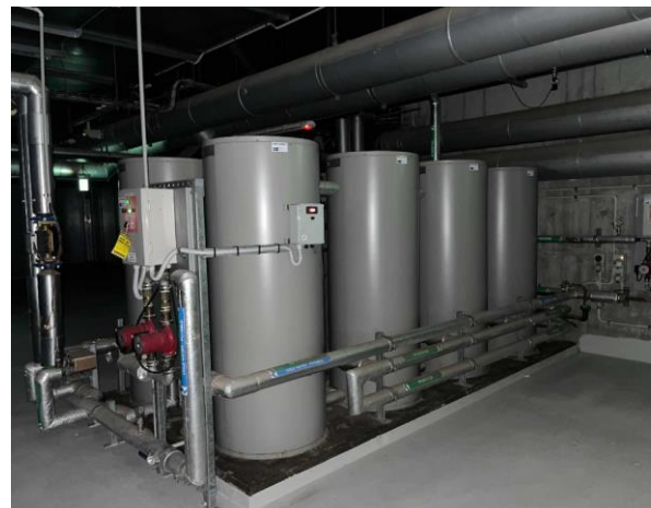
Line ID 12: Internal, L1, Plant Room, Throughout, Pipework, Internal Insulation - Suspected SMF
