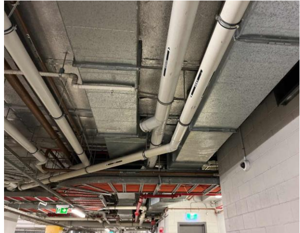
Line ID 24: Internal, Basement, Throughout, AC Ductwork, Insulation Material - Suspected SMF
