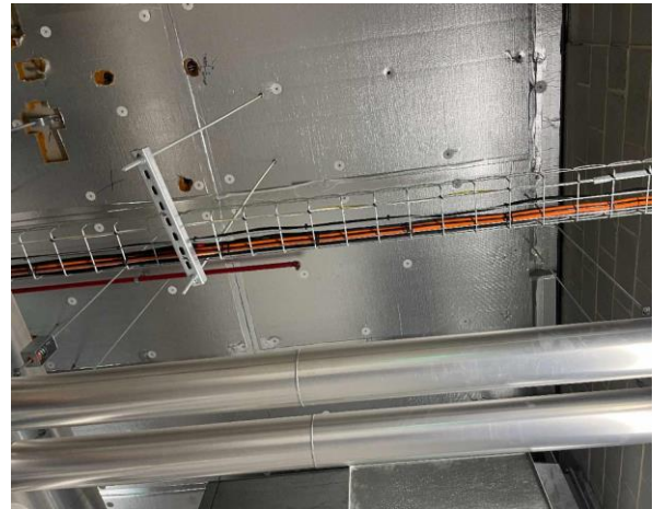
Line ID 14: Internal, L18, Generator Room, Ceiling, Insulation Material - Suspected SMF
