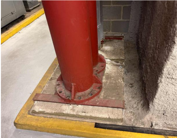
Line ID 1: Internal, L32, Plant Room, Base of Pipes, Around Insulation, Mastic Sealant - No Asbestos Detected
