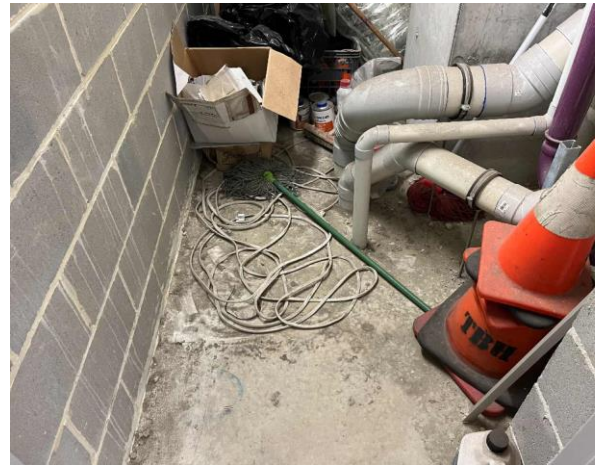
Line ID 8: Internal, L1, Small Plant Room, Floor throughout, Dust - Lead Detected (56mg/kg)
