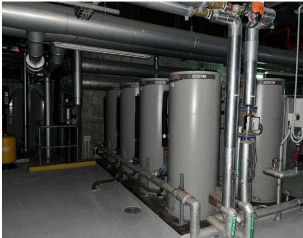
Line ID 13: Internal, L1, Plant Room, Within Hot Water Heaters, Insulation Material - Suspected SMF
