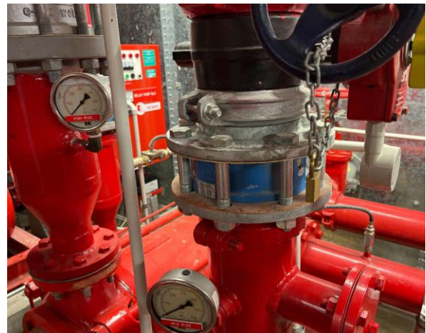
Line ID 6: Internal, Basement, Sprinkler Pump Room, Orange Gasket to Pipework, Gasket Material - No Asbestos Detected
