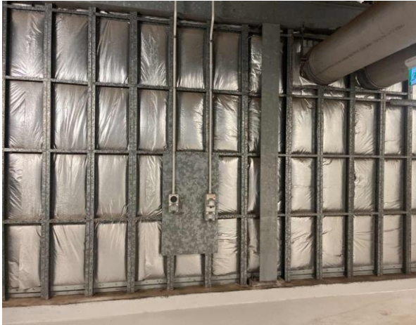
Line ID 20: Internal, L32, Plant Room, Throughout Walls, Insulation Material - Suspected SMF
