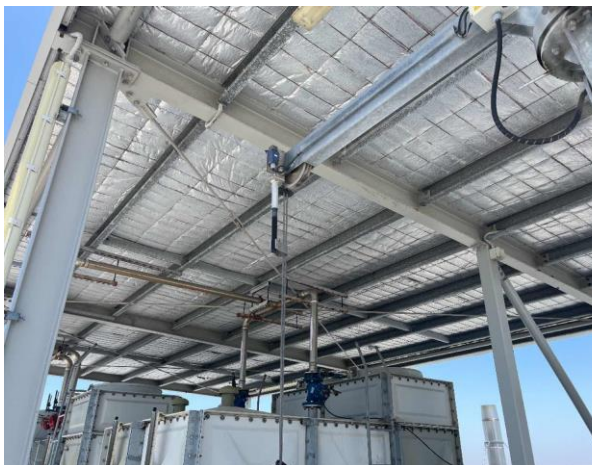
Line ID 11: External, Roof, Water Tank Area, To Ceiling, Insulation Material - Suspected SMF
