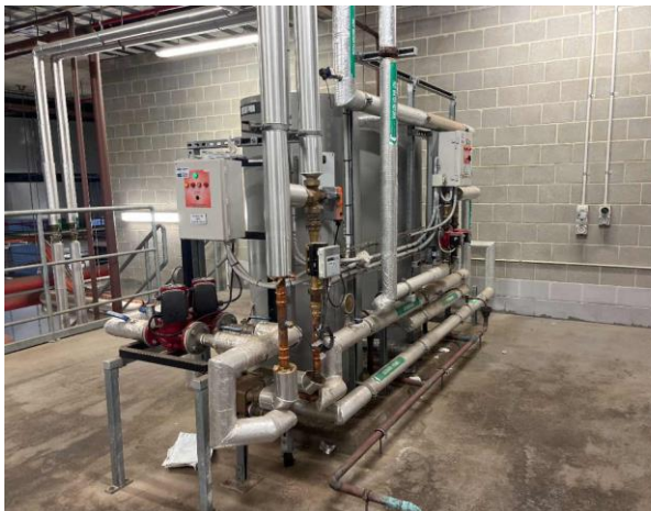
Line ID 15: Internal, L32, Mezzanine Area, Surrounding Pipework, Insulation Material - Suspected SMF
