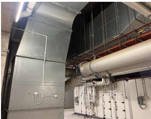
Line ID 17: Internal, L32, Plant Room, AC Ductwork, Internal Insulation - Suspected SMF
