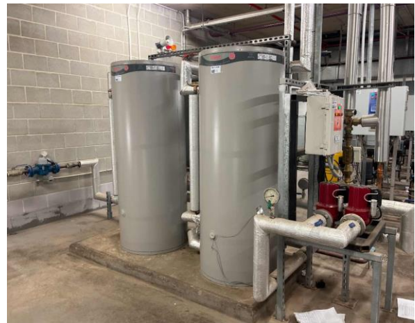
Line ID 16: Internal, L32, Mezzanine Area, Within Hot water Heaters, Internal Insulation - Suspected SMF
