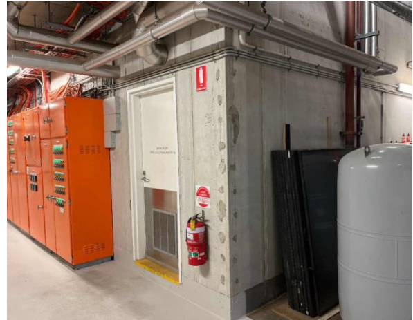
Line ID 2: Internal, L32, Plant Room, Boiler Room Walls, Fibre Cement Sheet - No Asbestos Detected
