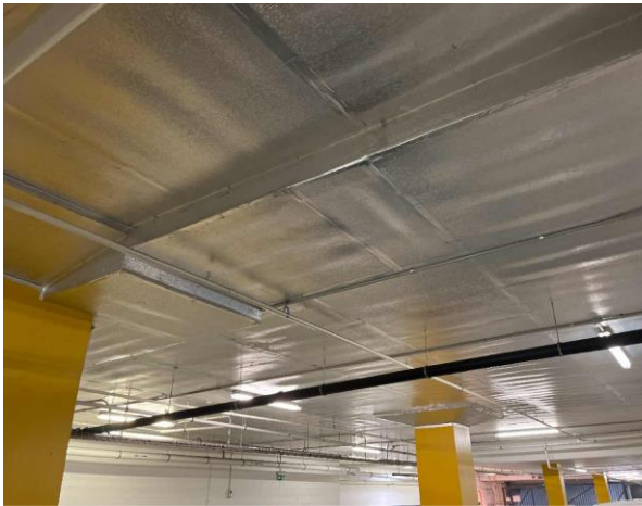
Line ID 25: Internal, Basement, Throughout, Ceiling, Insulation Material - Suspected SMF
