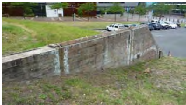
Figure 5.2 Remains of the lower brick walls of the eastern wall of the former foundry. (Source: GML 2010)
