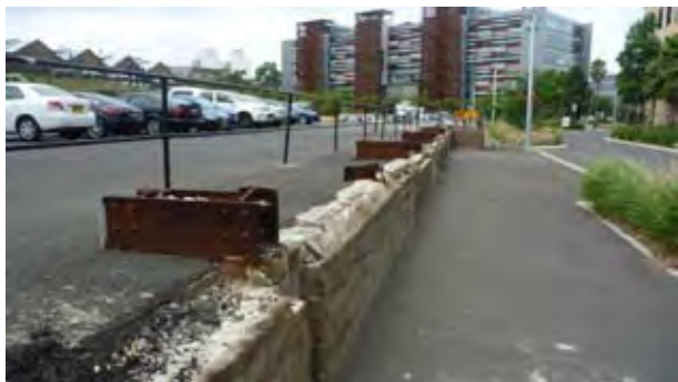
Figure 5.4 Brick footings from the southern wall of the former foundry. (Source: GML 2010)
