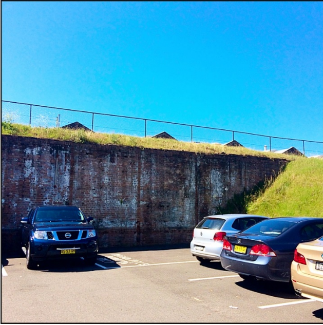
FIGURE 40: VIEW OF THE FABRIC OF THE REMNANT FOUNDRY WALL, NORTH, WITH LOCOMOTIVE ROOF VISIBLE IN BACKGROUND. (SOURCE: CURIO PROJECTS 2016)
