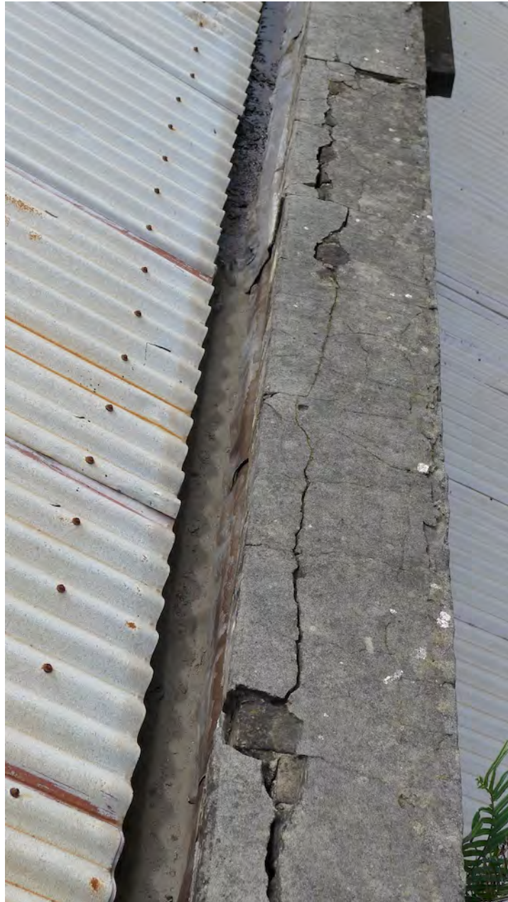
Figure 11 – Note that the breakdown of the render is uncovering underlying fractures of the sandstone coping.
