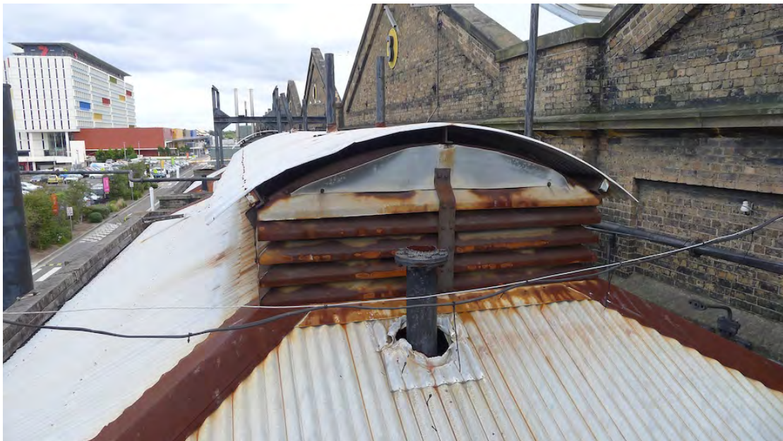
Figure 13 – The roof covering of the Bay 2 Annex. Note the rusting hip flashings, the damaged and corroded louvers, the distorted capping to the surmount and poorly flashed penetrations.
