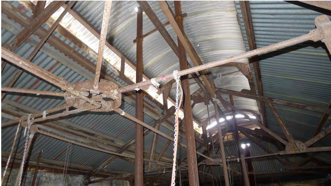
Figure 12 – Internal view of the roof structure of the Bay 2 Annex. Note the complex junction of tie rods at the hip apex.
