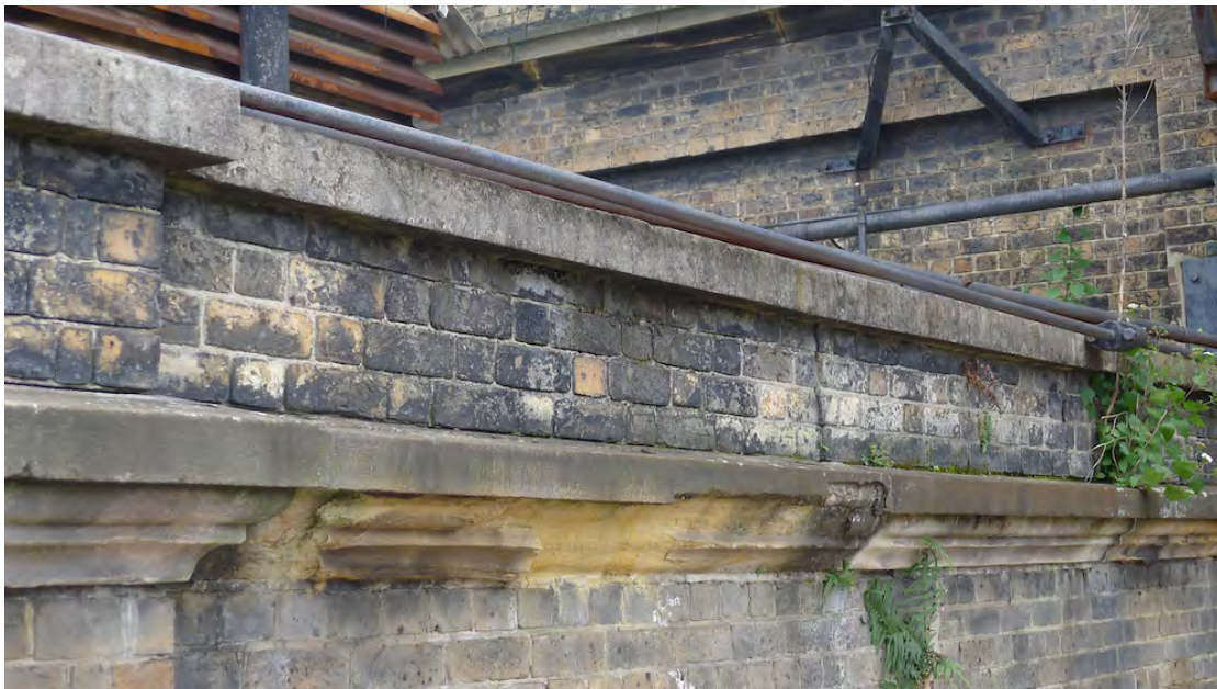
Figure 9 – Erosion of sandstone elements and plant growth on the Bay 2 Annex.
