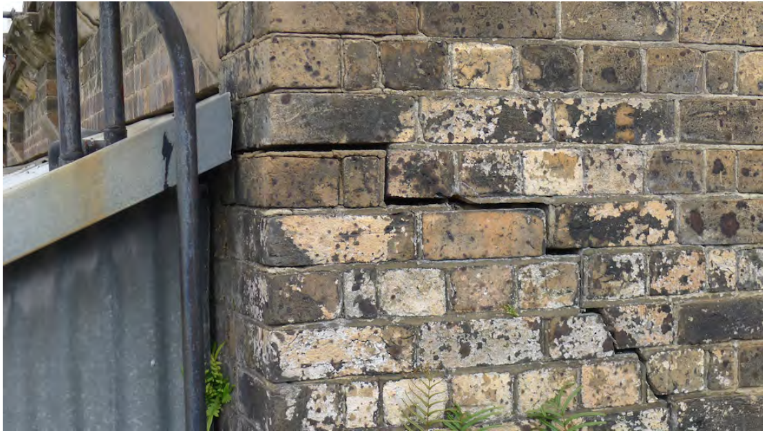
Figure 8 – Cracking of the brickwork caused by rust jacking.
