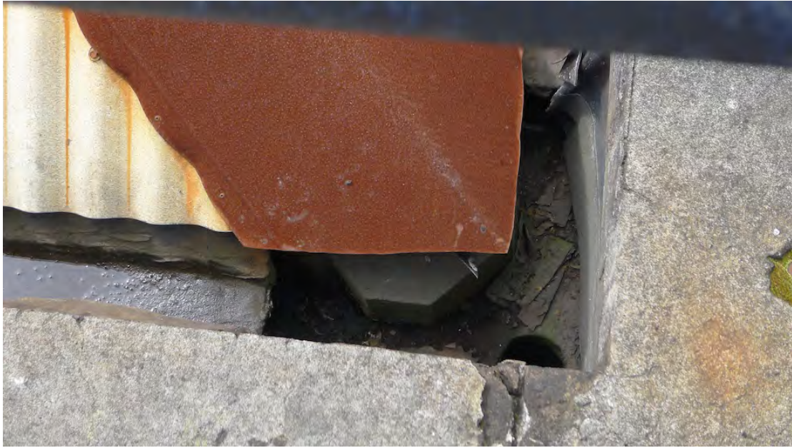
Figure 14 – Detailed photograph of the guttering of the Bay 2 Annex. Note the downpipe appears to discharge into a concealed downpipe. The associated plant growth would suggest the drainage line no longer functions and the surface water saturates the masonry.
