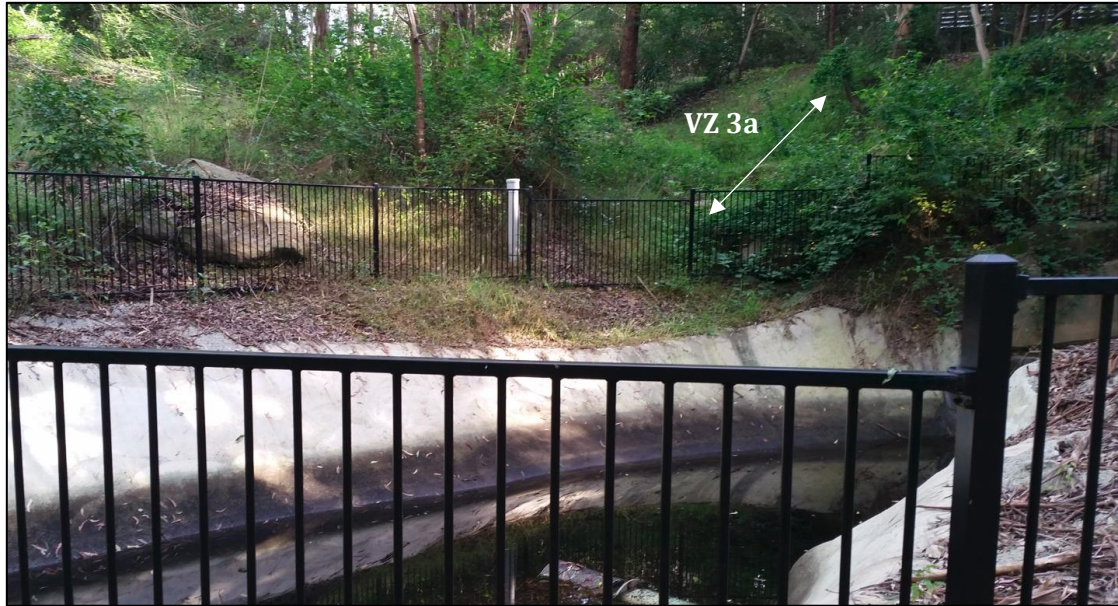
Figure 11: Vegetation Zone 3a above the detention basin to the south of the perimeter road. This clearly shows the battered nature of this zone, leading down from and supporting the road. Photo by E. Ashby, 20 th June 2014.
