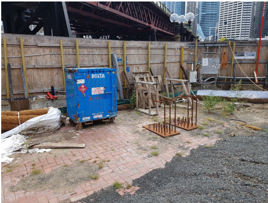
Photo 32: Flammable liquids cabinet near the north-astern corner of the site with a continuous particulate (PM 10 ) dust monitor to the right and Pymont Bridge in the background. 23/01/24
