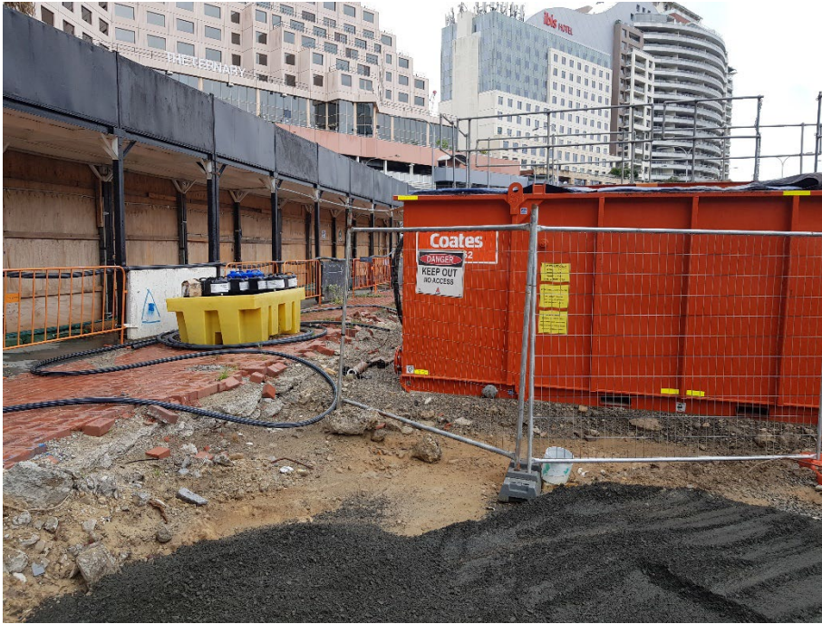
Photo 29: Part of the Dewatering Treatment Plant located near the south-western boundary. Water treatment chemicals stored on a pallet bund. Black acoustic matting visible on top of the generator unit for noise mitigation. Dark grey/black imported fill visible in the foreground. 23/01/24
