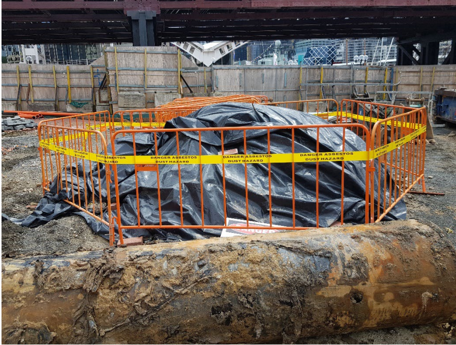
Photo 35: A stockpile of asbestos contaminated soil located in the northern part of the site. 23/01/24
