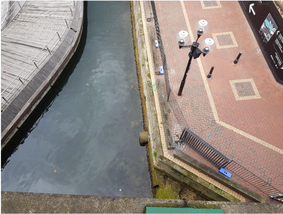
Photo 3: View from Pymont Bridge looking at the northern section of the Boardwalk and Darling Harbour. 16/01/24
