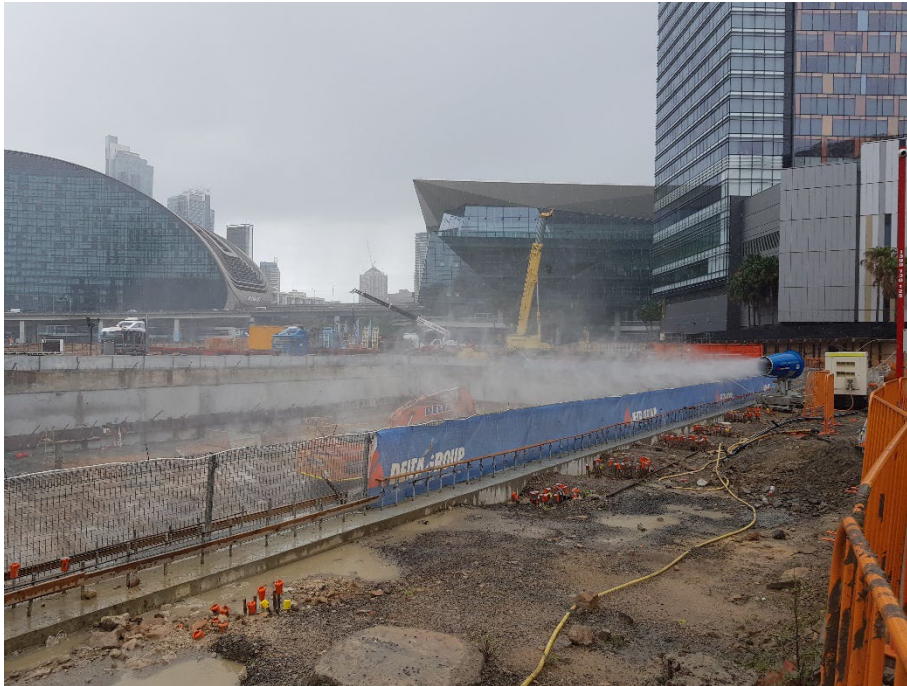
Photo 21: View from the western side of the site looking to the southeast across the basement excavation. A large water misting cannon was in use for dust mitigation. 23/01/24
