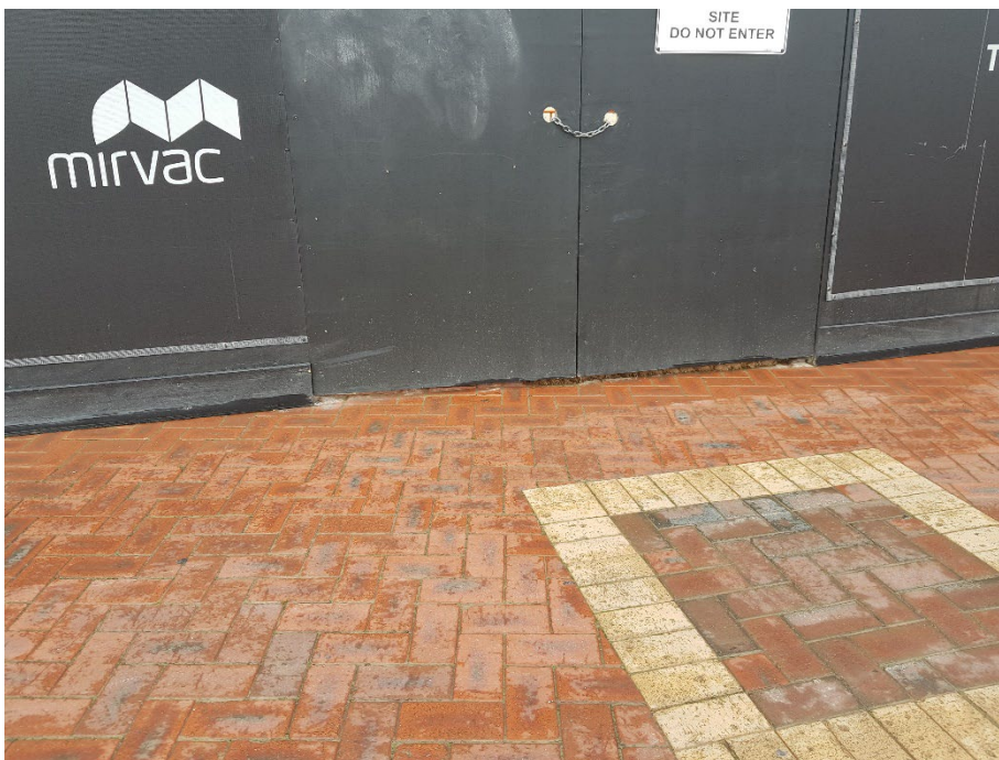
Photo 8: A gate in the hoarding along the boardwalk where the coir log is visible in the gap beneath the gate. 16/01/24
