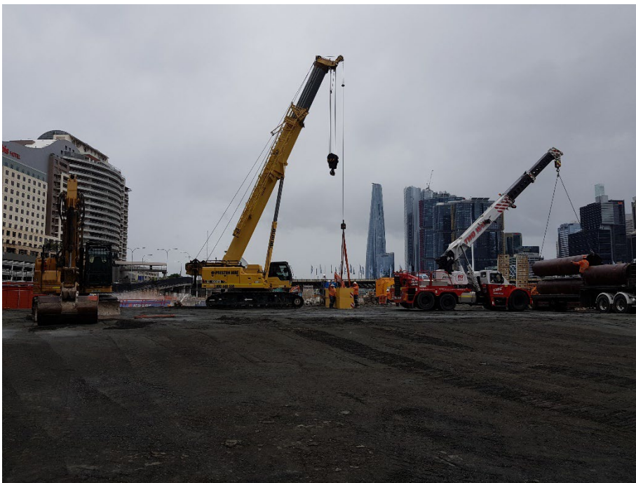
Photo 288: The plant (cranes) that arrived earlier in the morning outside construction hours. Dark grey/black imported fill spread across the southern portion of the site. 23/01/24
