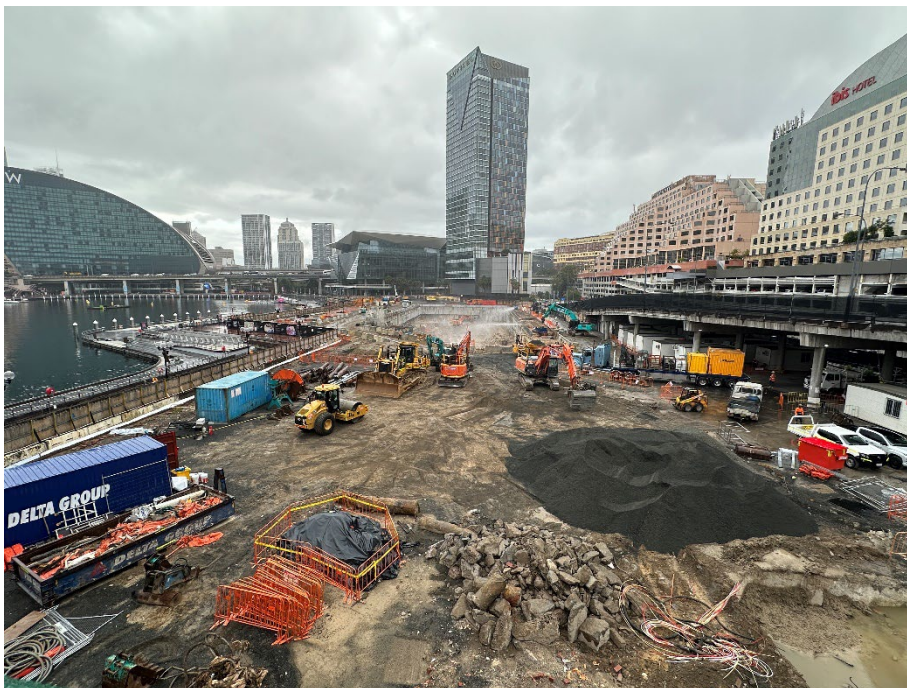
Photo 40: View from Pyrmont Bridge looking south across the site. Dust mitigation in operation. Covered and fenced soil stockpile containing asbestos in the foreground, as well as a larger stockpile of imported material. 23/01/24
