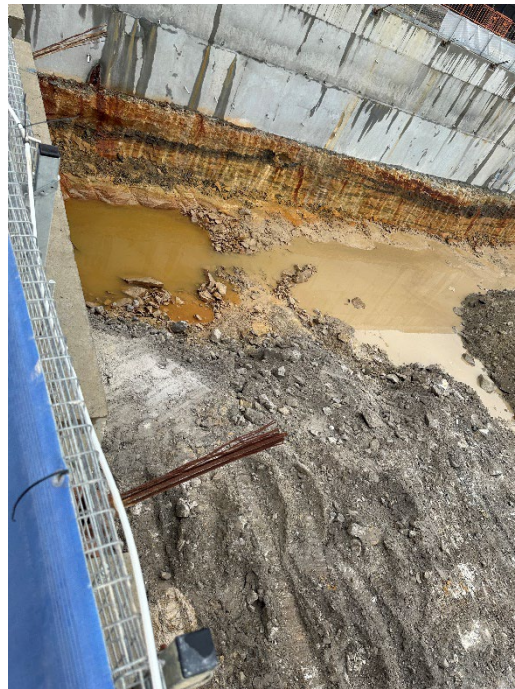
Photo 34: Water collected in the south-western corner of the basement excavation. 23/01/24
