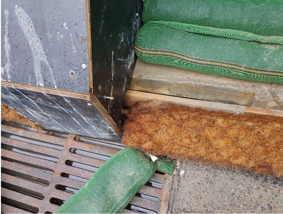
Photo 17: Closer view of the sediment controls and geotextile mesh protecting the drain. 23/01/24
