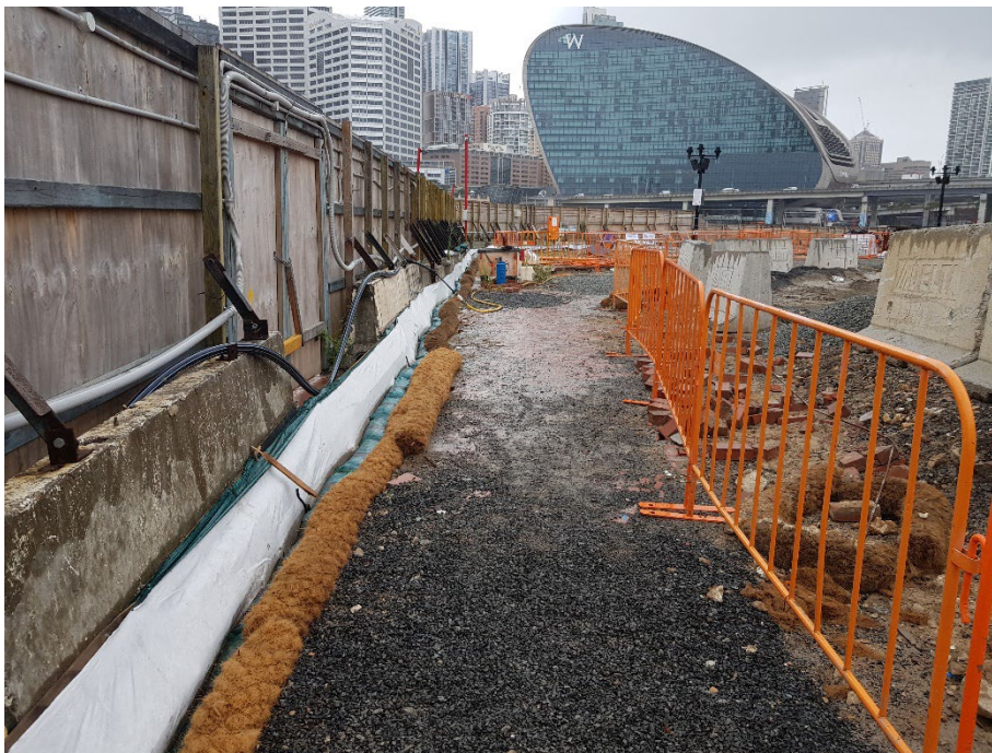
Photo 24: View to the south along the eastern site boundary hoarding showing the sediment controls that were maintained during the preceding week. 23/01/24
