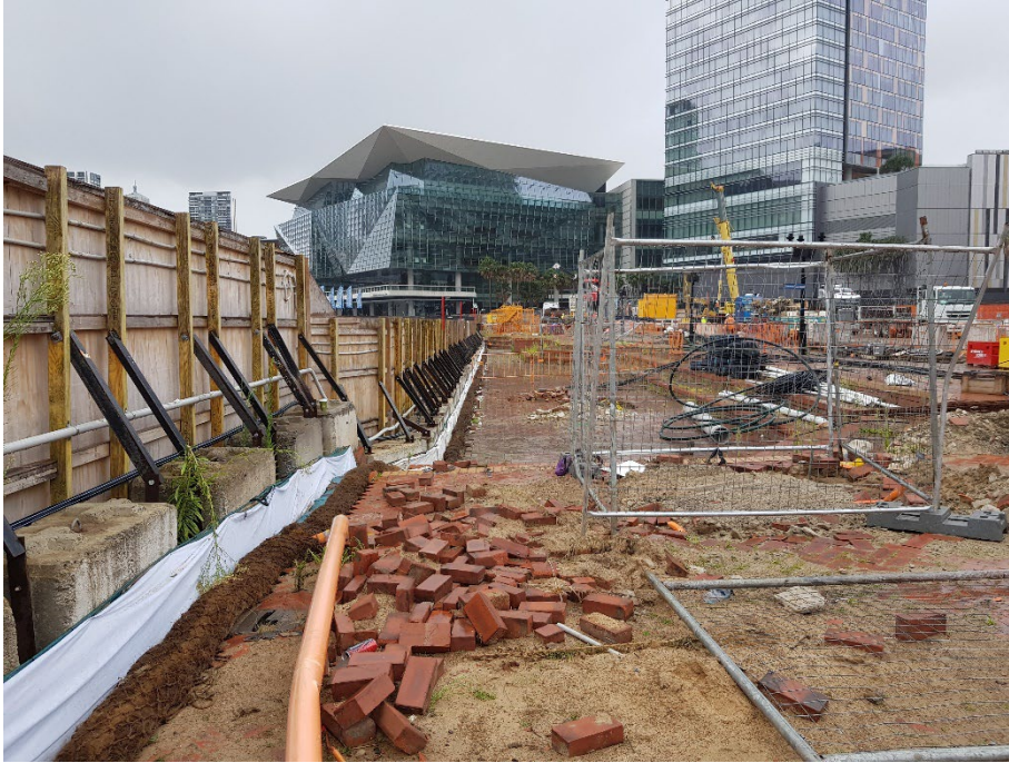
Photo 25: View to the south along the eastern site boundary hoarding showing the sediment controls that were maintained during the preceding week. The site level is lower along some parts of the eastern boundary. 23/01/24
