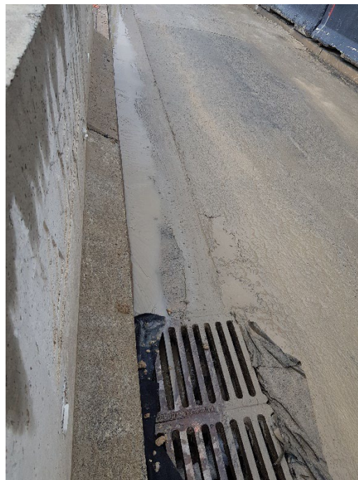
Photo 20: A street stormwater drain that the truck wheel wash drains towards, which was missing a geotextile sausage to prevent sediment entering the drain. 23/01/24
