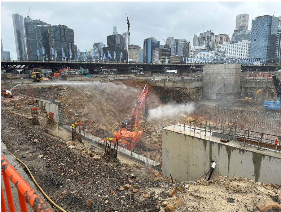
Photo 22: View from the western side of the site looking to the northeast across the basement excavation. A smaller water spray cannon was in use for dust mitigation. 23/01/24
