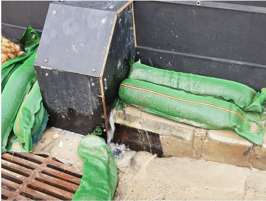
Photo 15: Additional sediment controls were placed against the hoarding and the volume of water had decreased and appeared clearer. 09:49 16/01/24
