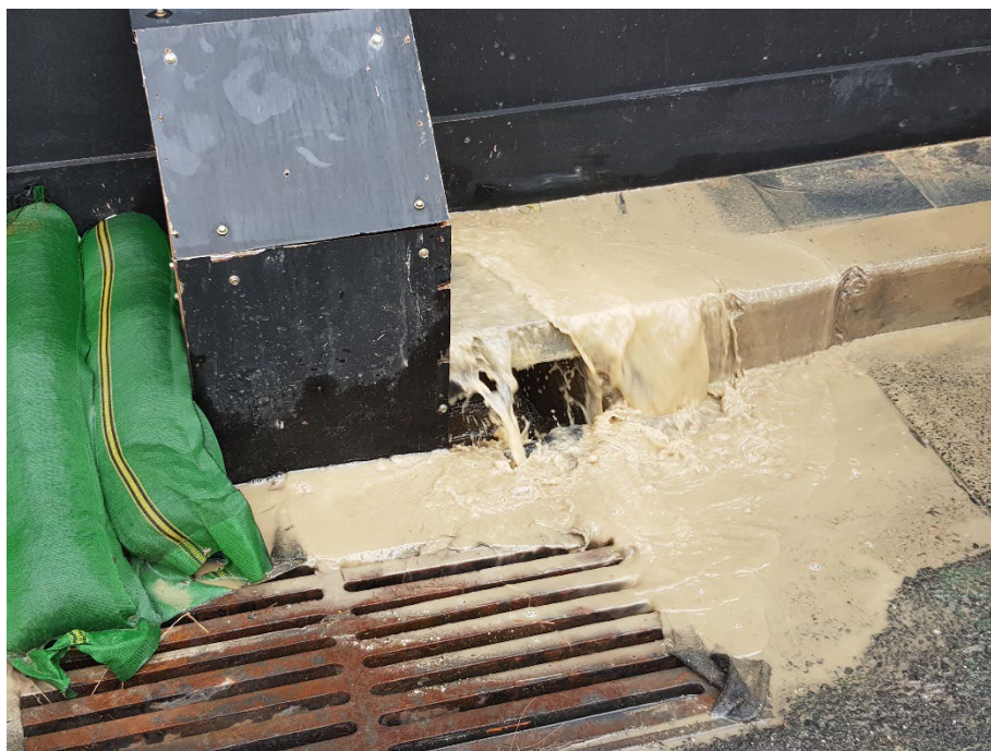
Photo 14: Sediment release from the site beneath the hoarding due to a burst water hose. 09:45 16/01/24
