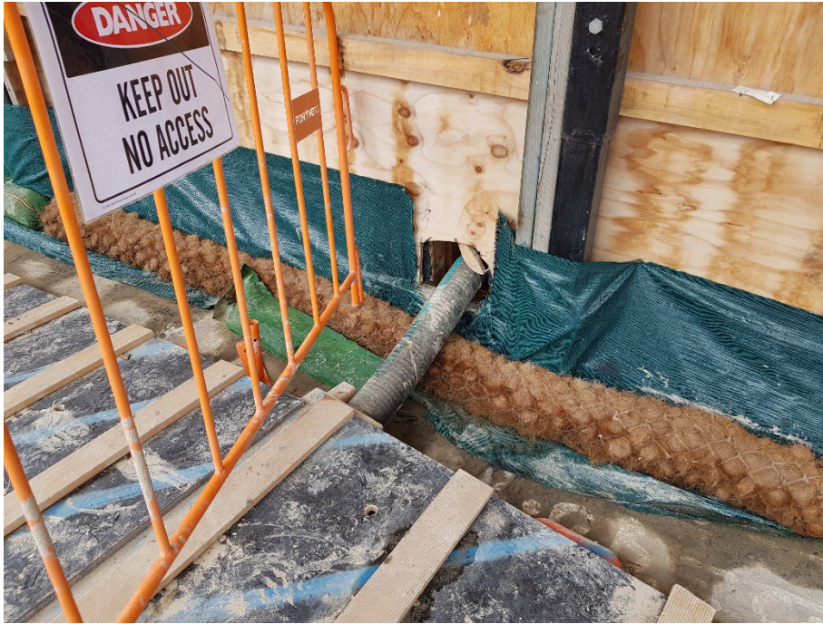
Photo 31: The discharge hose line for the Dewatering Treatment Plant, in the vicinity of where the burst hose and sediment release occurred on 16/07/24. The sediment control have been replaced. 23/01/24
