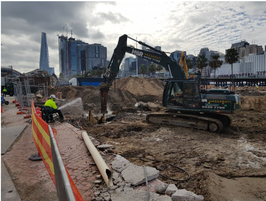
Photo 26: Worker directing water spray over the demolition work area. Looking towards the northeast.
