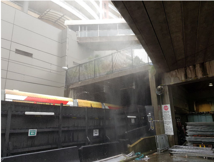
Photo 21: Water misting for dust suppression along the western boundary adjoining the light rail. Hoarding protects the light rail from site activities.
