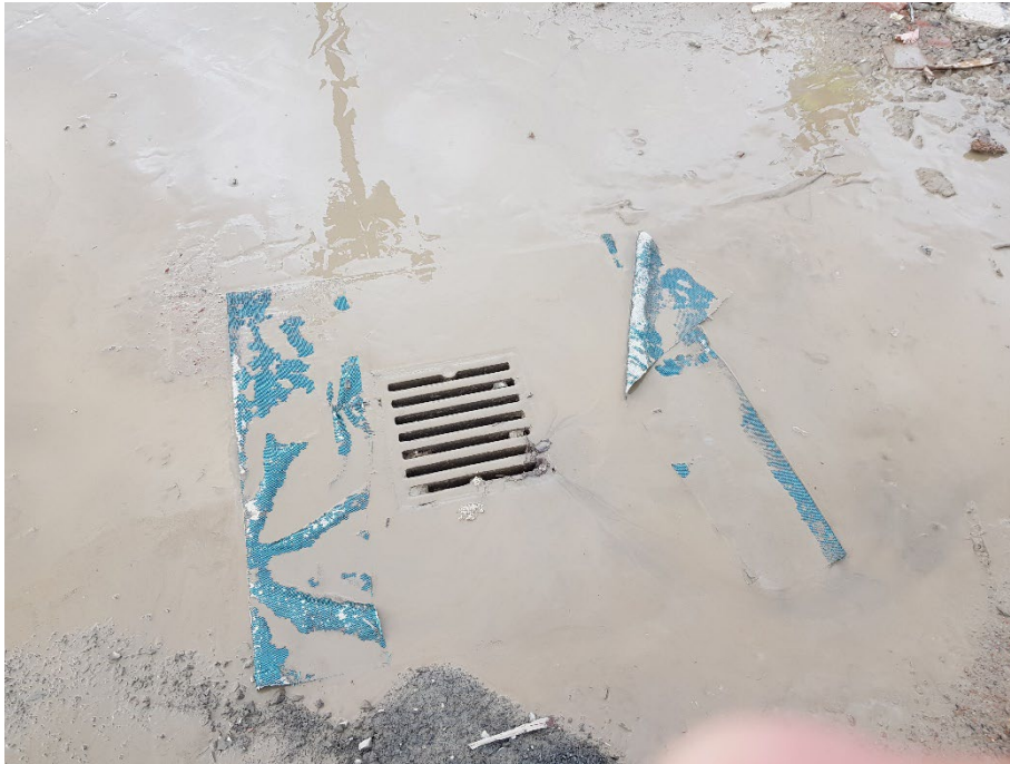
Photo 15: Geofabric lining in a stormwater drain located within the southern portion of the site.
