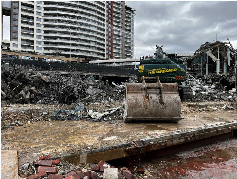
Photo 27: Water spraying from hose over the demolition work area. Looking towards the northwest.
