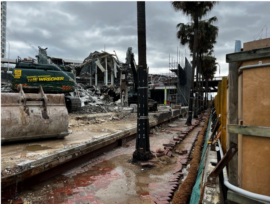
Photo 28: Water spraying from hose over the demolition work area. Also the likely source of the water seeping under the site boundary fence shown in Photos 5 and 6.
