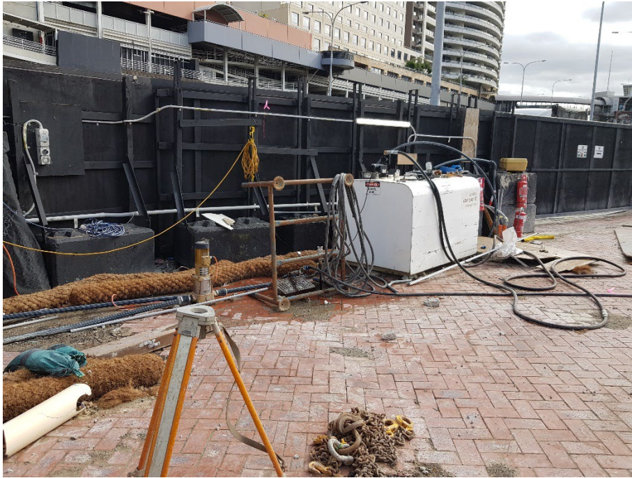
Photo 23: Self-bunded diesel tank located near the site entrance.
