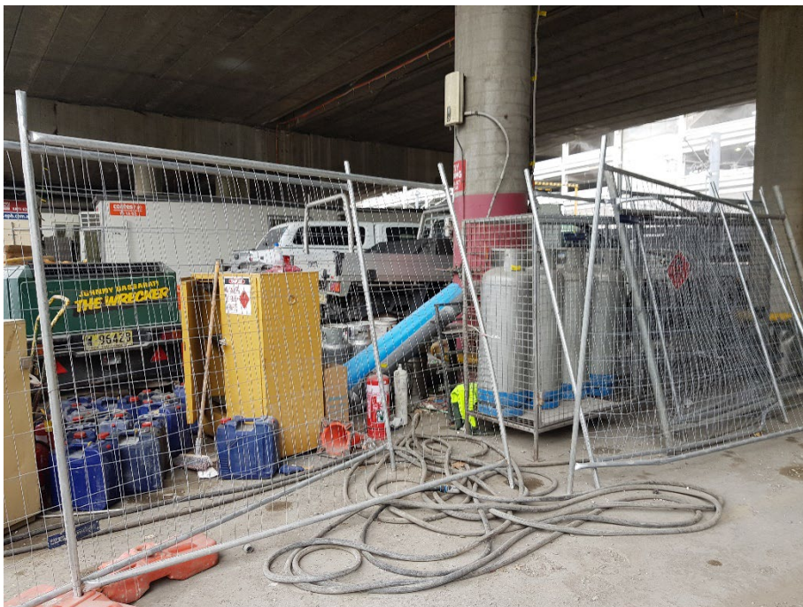
Photo 24: Chemical storage area under the Darling Drive overpass next to the site offices, noted by the Auditors during the site visit as needing improvement.
