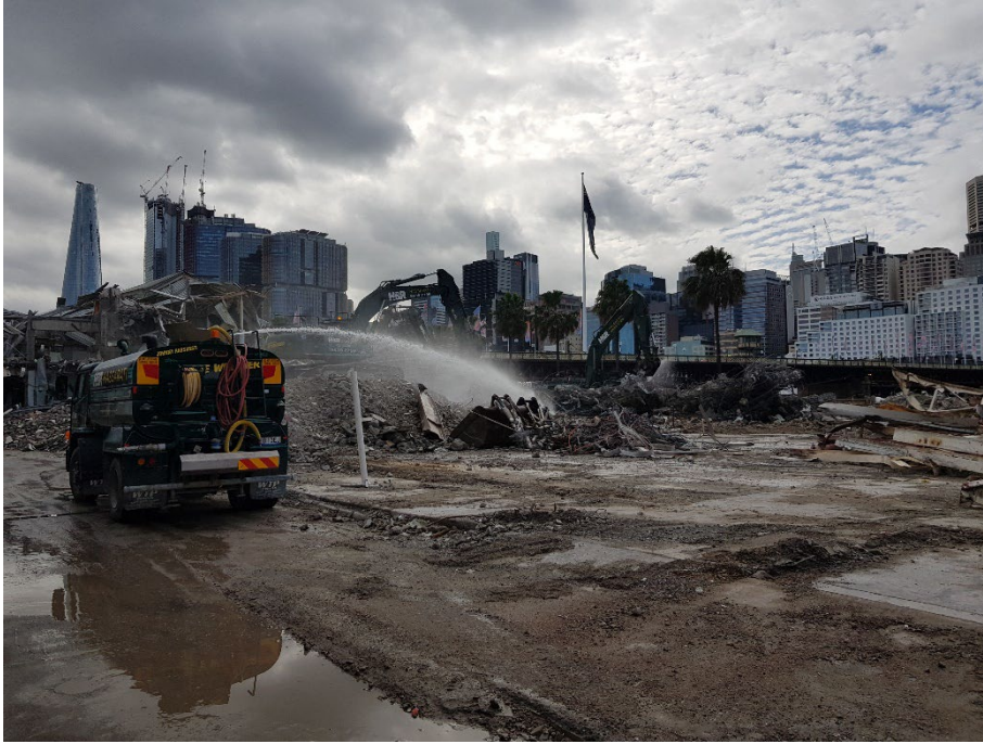
Photo 25: Water cart in operation during demolition in the central portion of the site. Looking towards the northeast.
