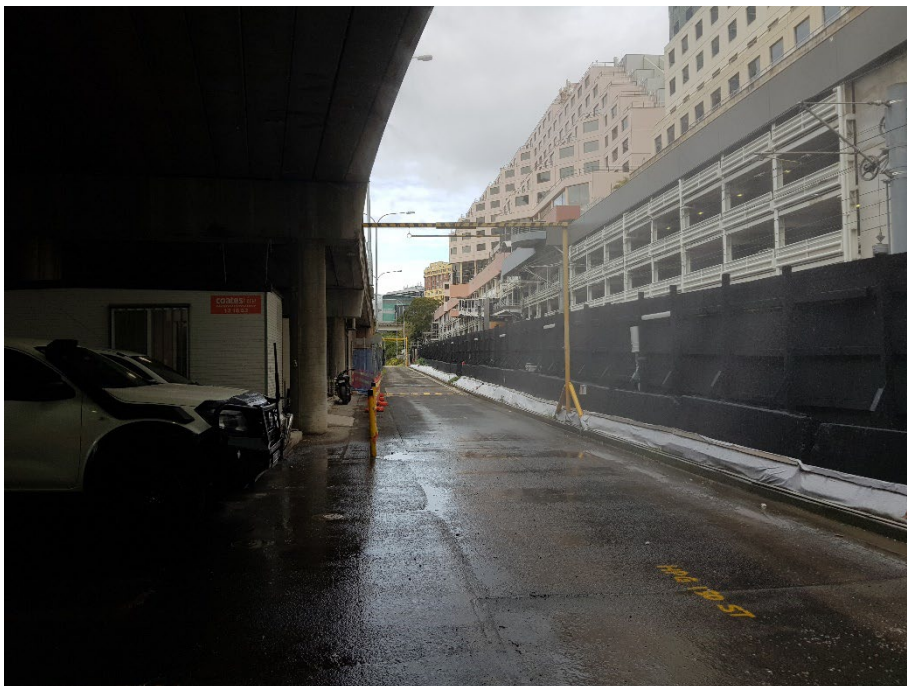
Photo 22: View to the south along the western vehicle exit looking towards Darling Drive roundabout. Water misting for dust suppression. Hoarding on the right protects the light rail from site activities.
