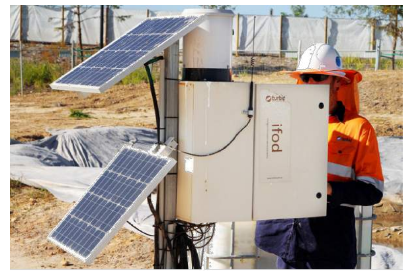
iFOD FLOW DOSING UNIT (CUSTOM BUILT)
